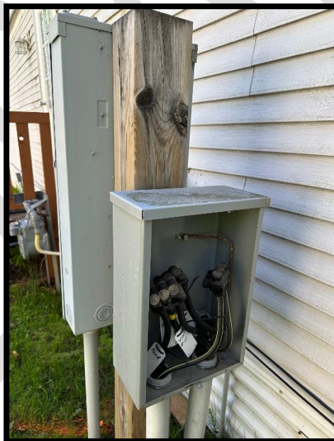
Figure 2: Junction Box with Meter Base
