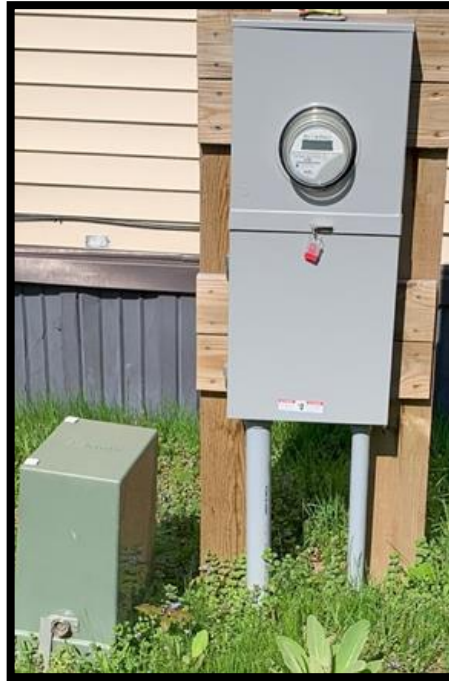
Figure 1: Ped with Meter base.
