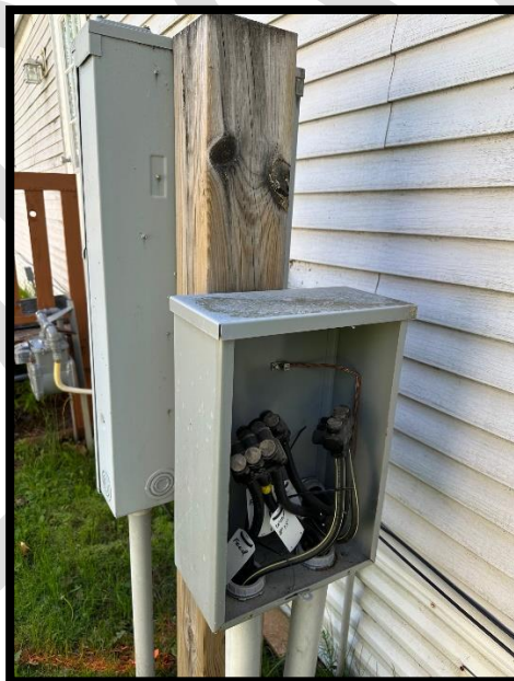
Figure 2: Junction Box with Meter Base
