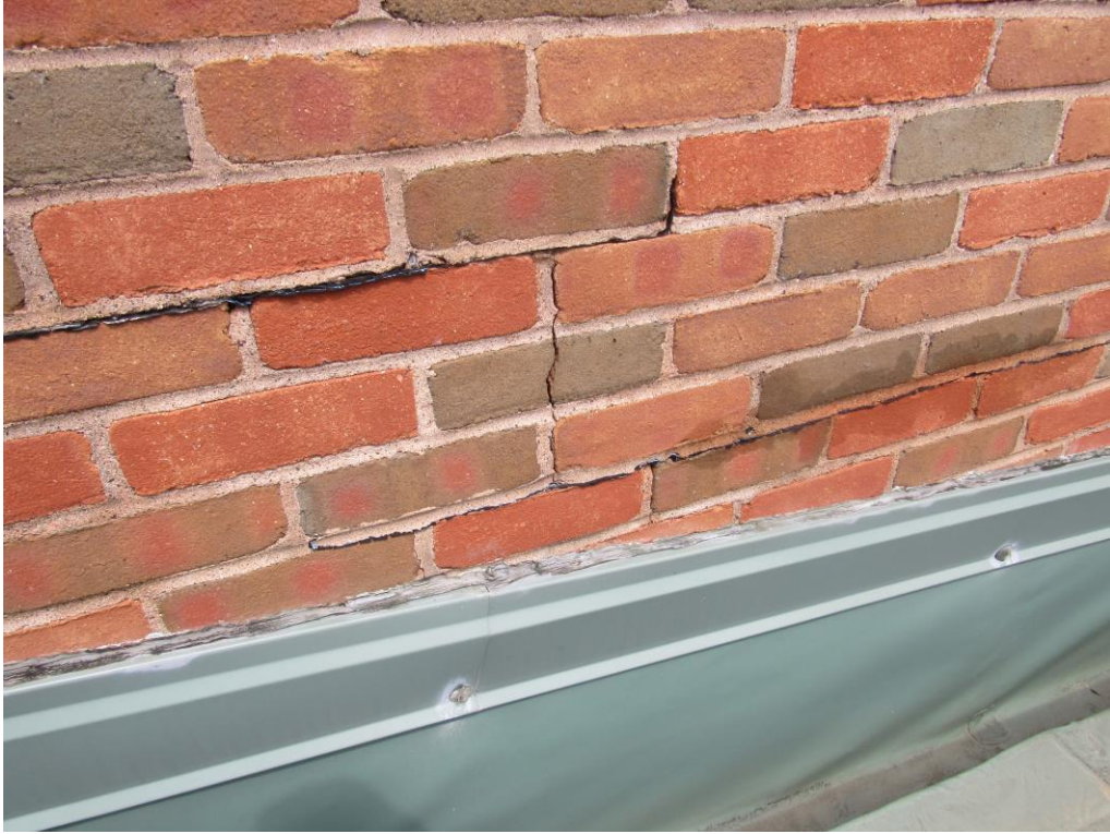
Photograph 16 – Brick crack around through wall flashing details.
