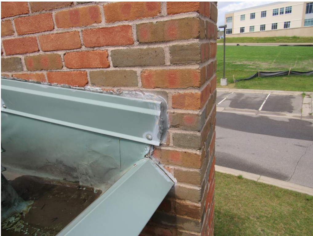
Photograph 27 – Failed sealants at metal flashings.
