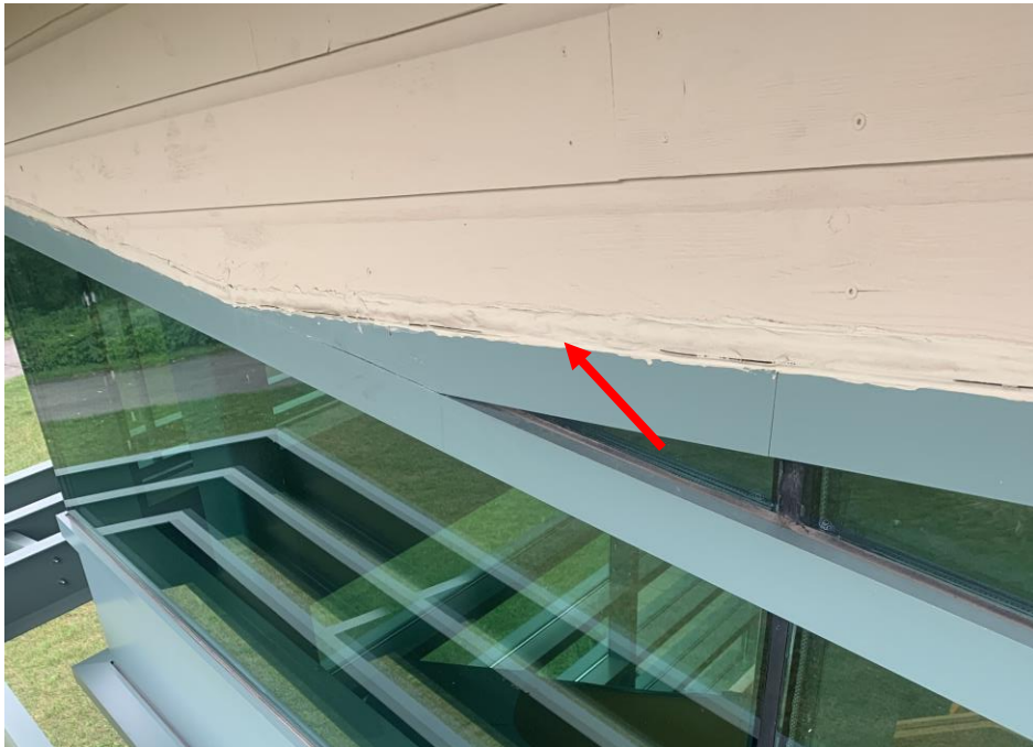
Photograph 25 – Sealant installed at window head/base of siding, with failures observed.
