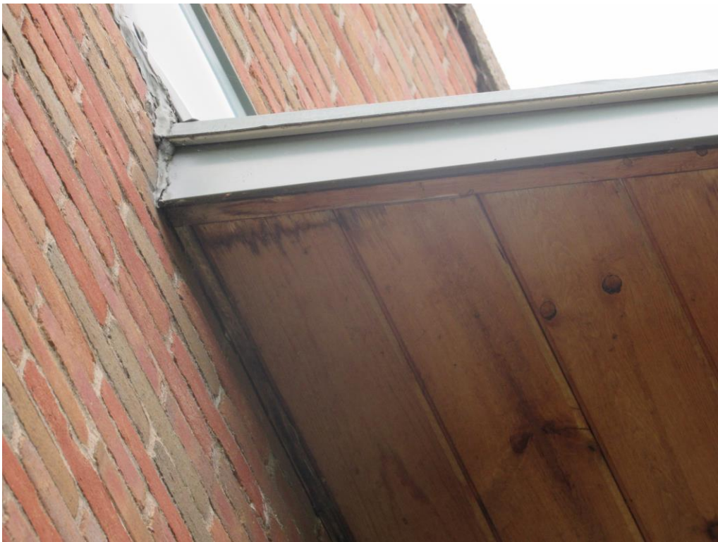
Photograph 17 – Water stains at a wood soffit.
