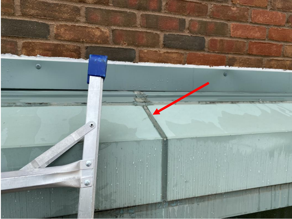
Photograph 5 – Joint above window head, note failed sealant, testing location is noted by arrow.
