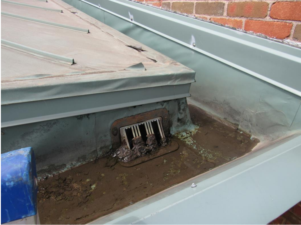
Photograph 30 – Roofing at the north roof elevation, with peeled terminations at the corner.
