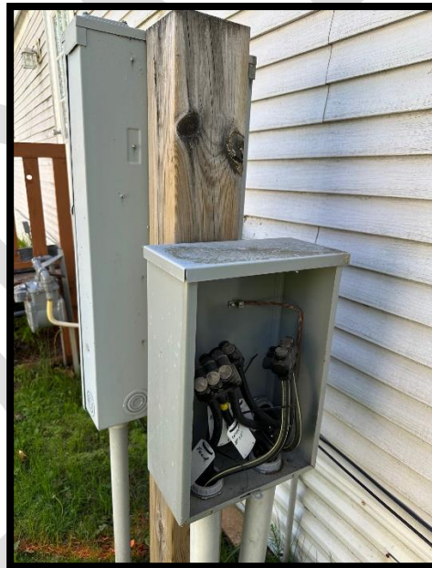
Figure 2: Junction Box with Meter Base
