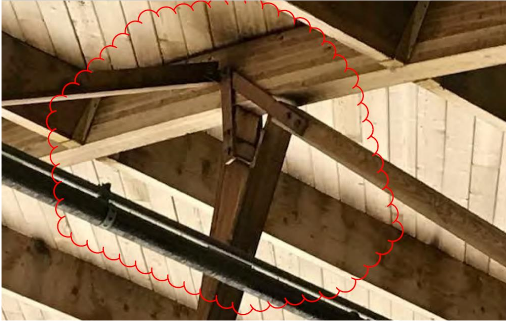
Picture of Failed Truss Member
