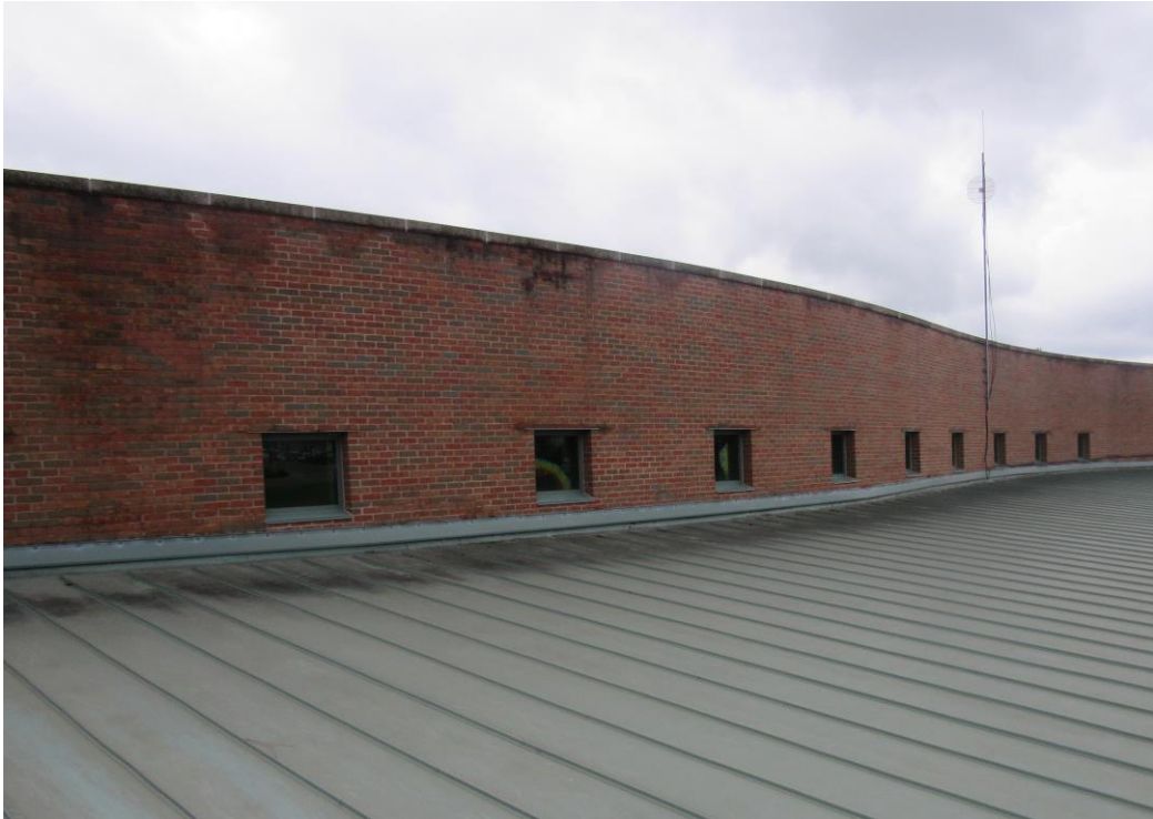
Photograph 13 – Water-stained masonry wall (north facing).
