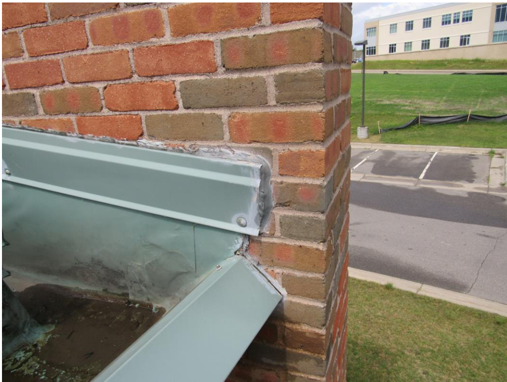
Photograph 27 – Failed sealants at metal flashings.
