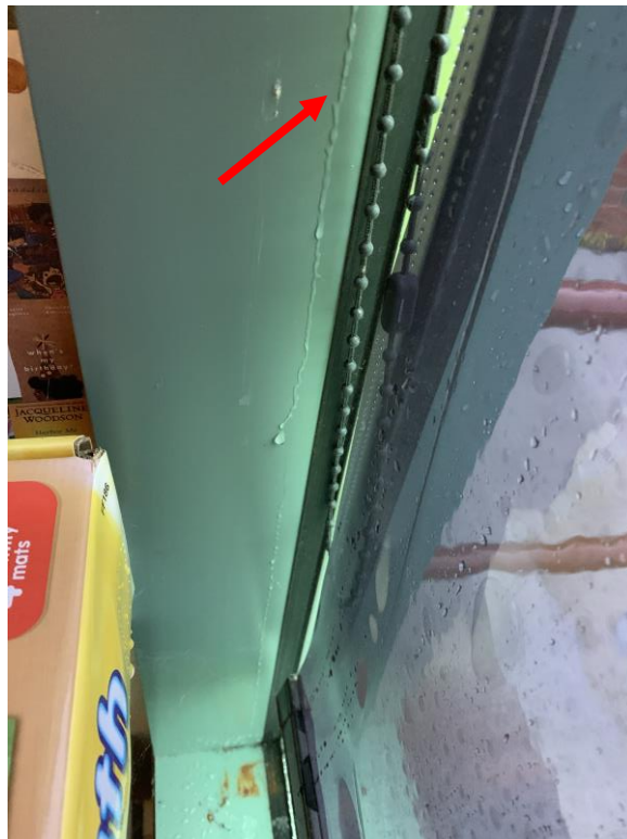
Photograph 8 – Leak location at the office window.
