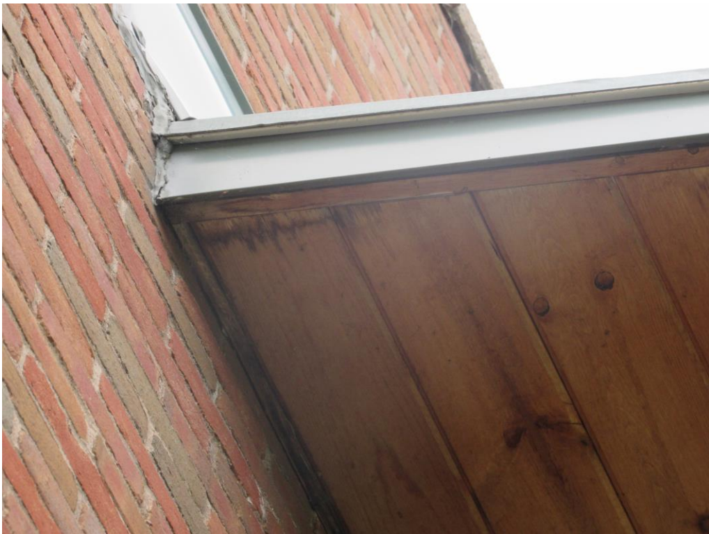
Photograph 17 – Water stains at a wood soffit.
