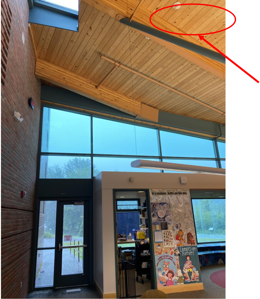
Photograph 9 – Reported leak location at the ceiling near the east entry doors.
