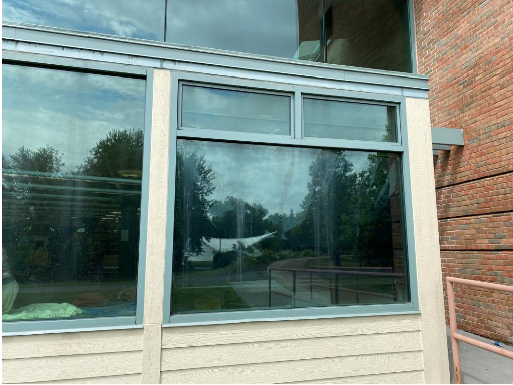
Photograph 7 – Office window with leaks reported at the interior jamb.
