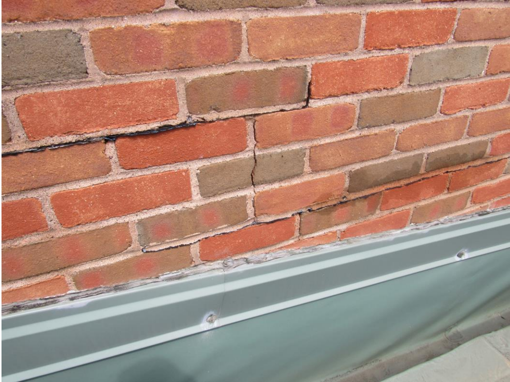
Photograph 16 – Brick crack around through wall flashing details.
