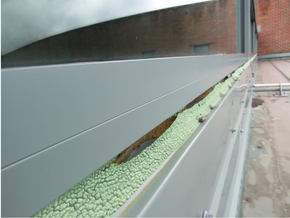
Photograph 24 – Failed sealant at a windowsill joint.
