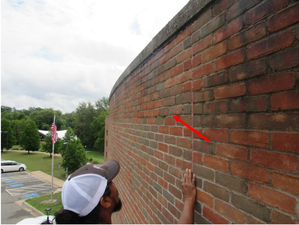
Photograph 14 – Water-stained masonry with cracking at bed joint. Moss formation is also noted.
