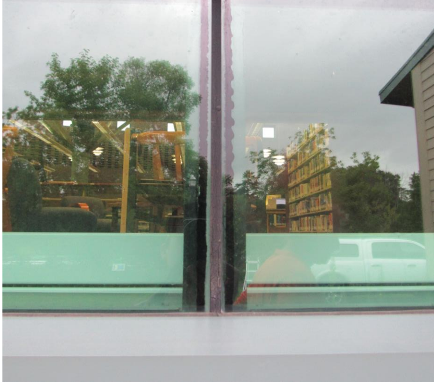
Photograph 18 – Cracking sealant at a window assembly.
