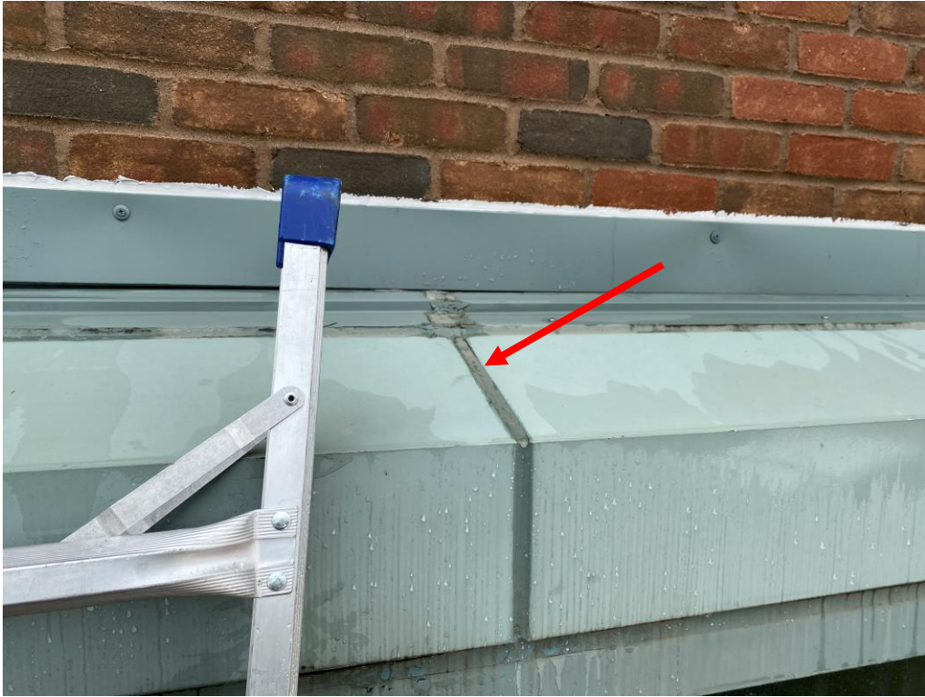
Photograph 5 – Joint above window head, note failed sealant, testing location is noted by arrow.
