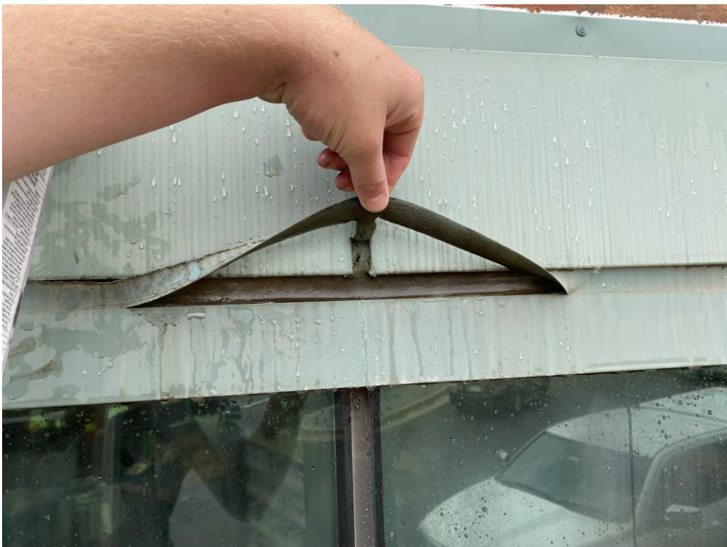
Photograph 6 – Failed sealant at joints in the bumpout window overhang assembly.
