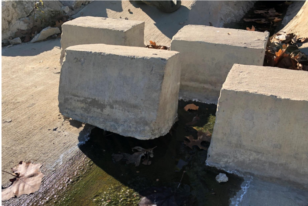
Photo 7: Any additional photos to support inspection (example, loose baffle block)
