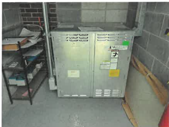
ELEVATOR OPERATING EQUIPMENT
