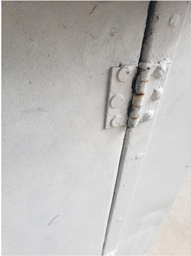
Book Return front door rusted completely from hinges
