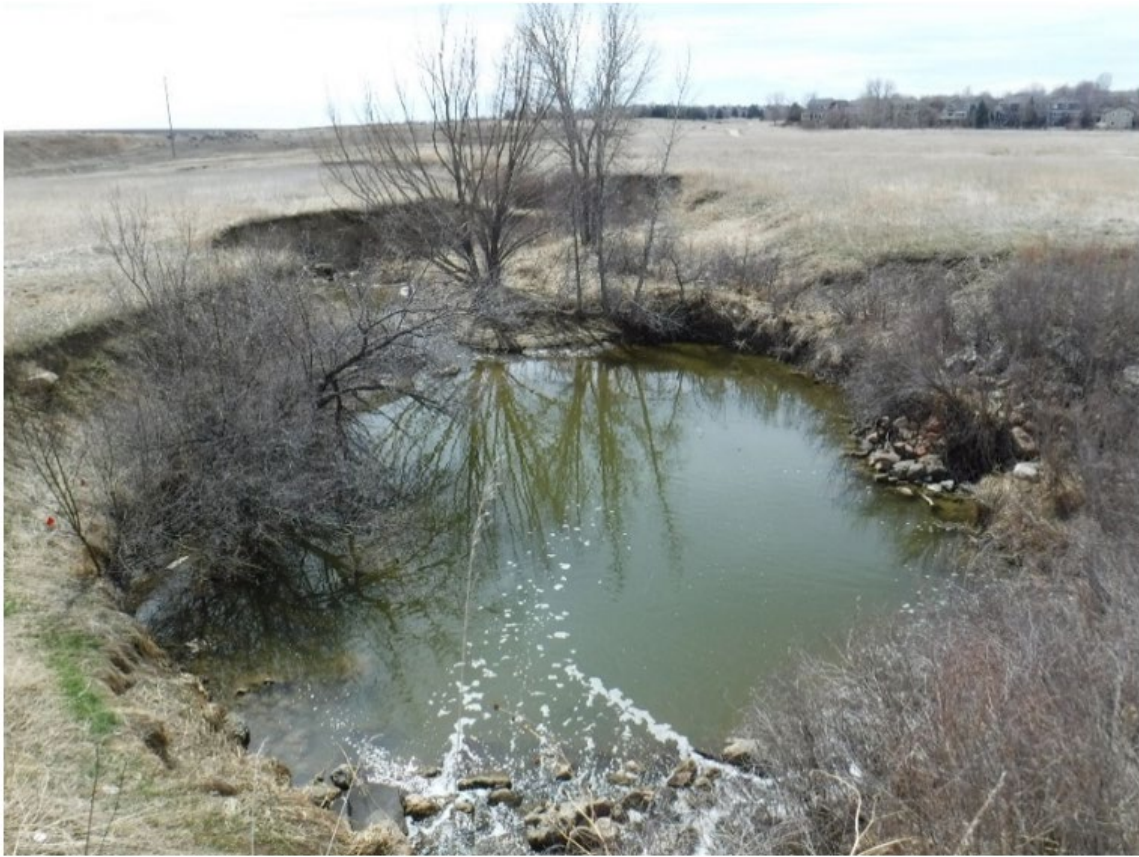
Photo 1. End of culvert looking south with four-ft deep scour pool and elevation drop (no fish passage)
