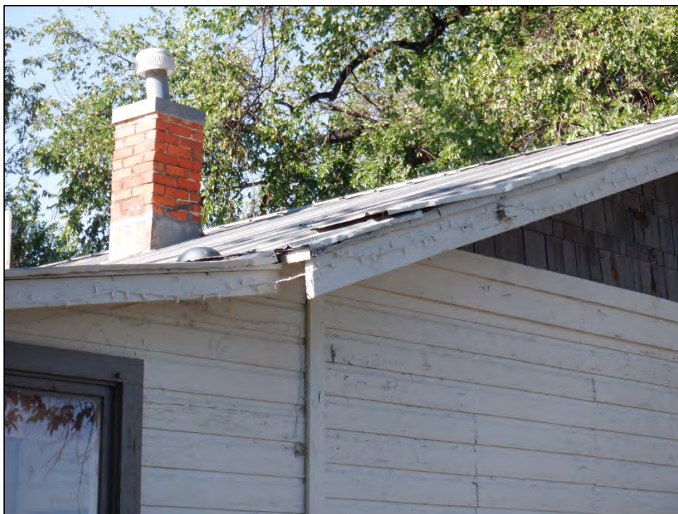
Figure 8: Feature 1, close up of loose roof panel, view southwest (Image #589, RLS 8/23/2022).
