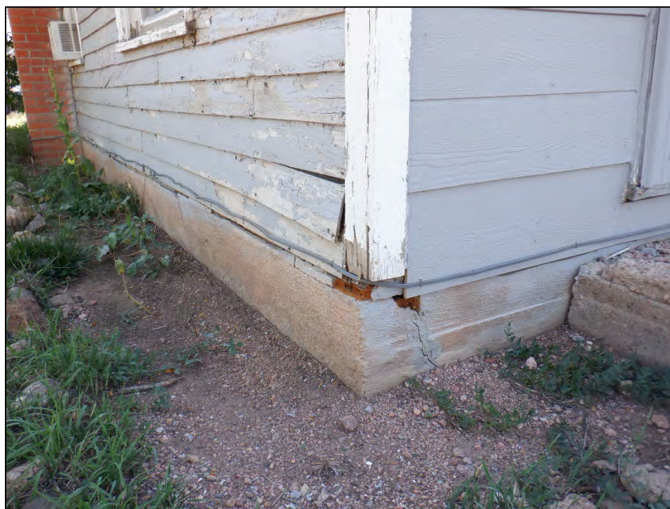
Figure 6: Feature 1, condition of northwest corner (Image #621, RLS 8/23/2022).
