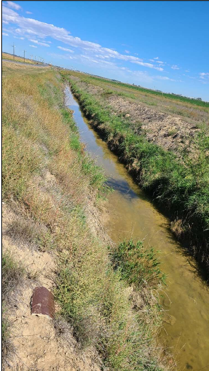
Photo 13. Timberline Road North – Segment 2: Facing north, the Number 8 Canal, parallel to Timberline Road (segment 2). Channel had steep vegetated banks which were eroding in areas. The canal continues south where it eventually drains into the Larimer and Weld Canal.
