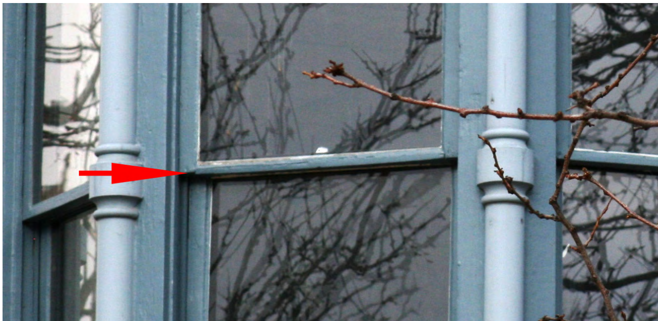
Image 20: Window 002-11, note meeting rail slipping down
