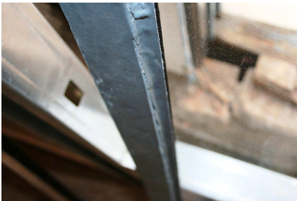
Image 13: Note the concave surface of the glazing compound. This is less effective at shedding water and does not replicate the historic appearance
