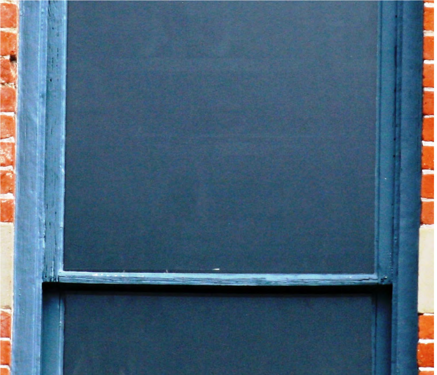
Image 21: Window 002-21 deterioration at the upper sash stiles and meeting rail left untreated
