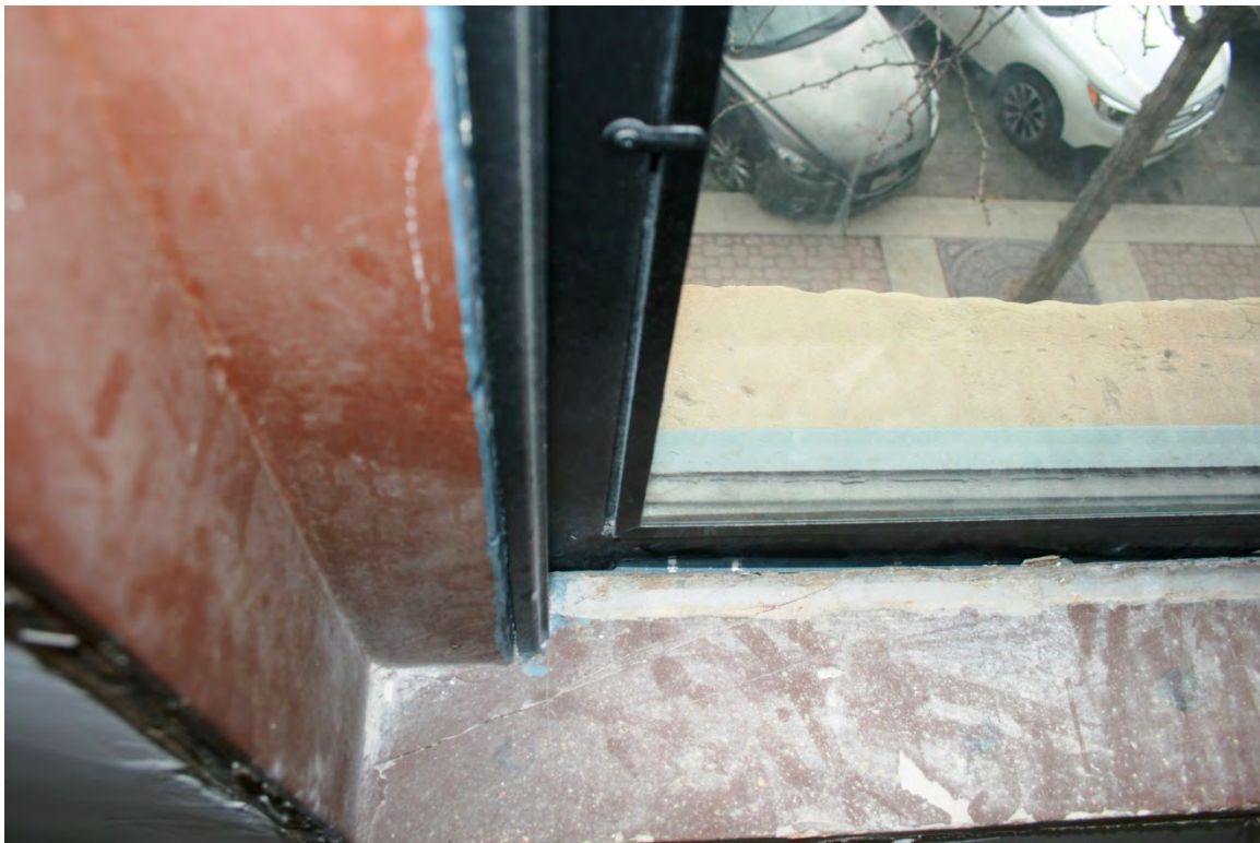
Image 9: Glass panel is slipping. Fit is loose
