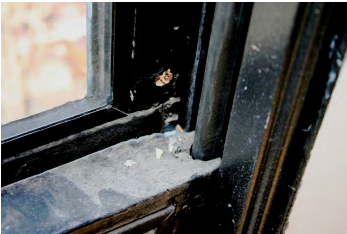
Image 11: Note flaking paint
