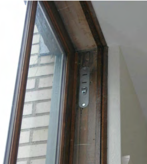
Image 3: Pullman balance installed in place of a window pulley. Photo courtesy of the Pullman website
