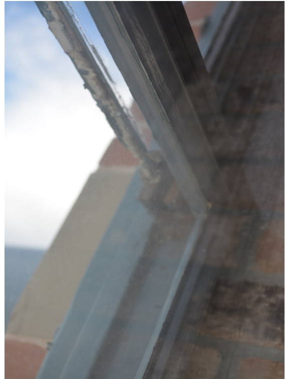
Sash With The Missing Check Rail
