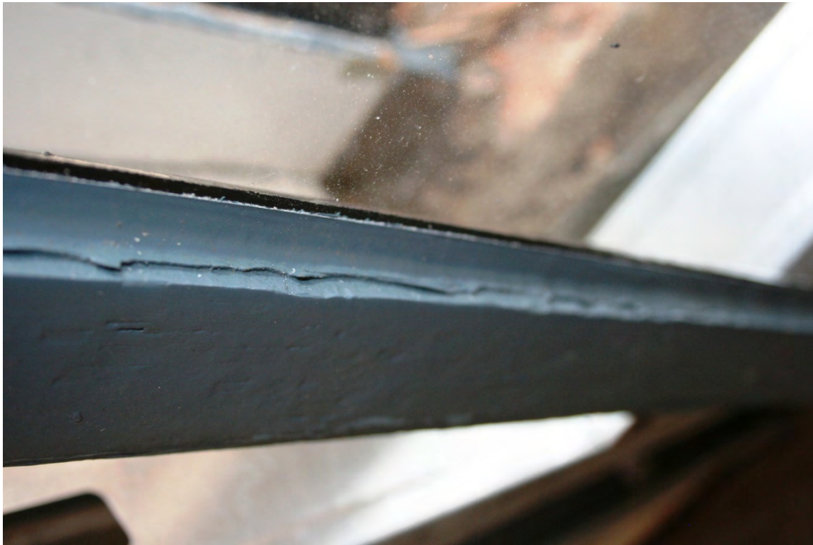
Image 14: Note how the new glazing compound does not come up to the edge of the bed and has a ragged edge
