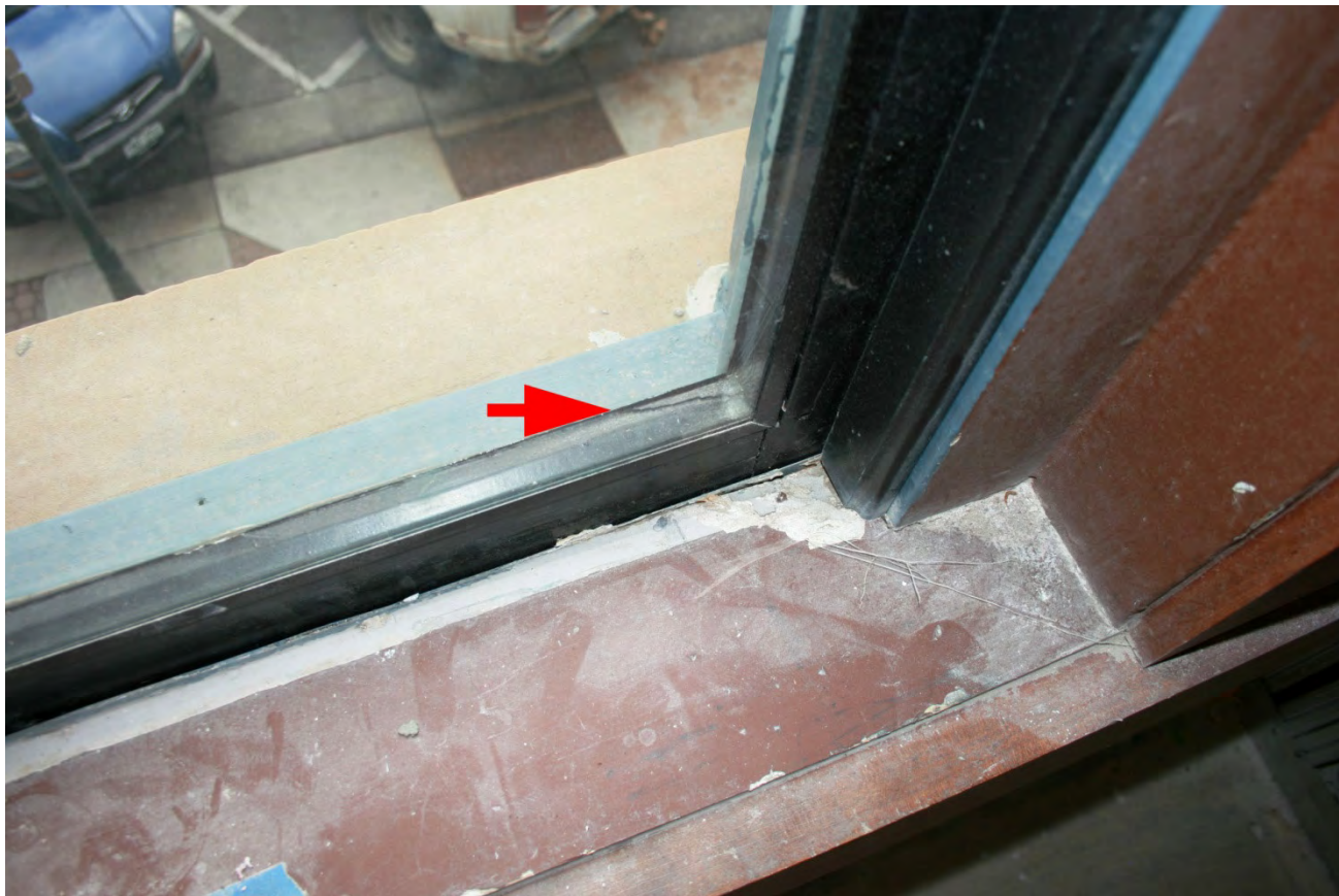
Image 19: Window 002-6, note crack in lower rail
