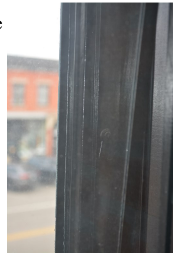
Tab Not Engaged, RDG is Loose
