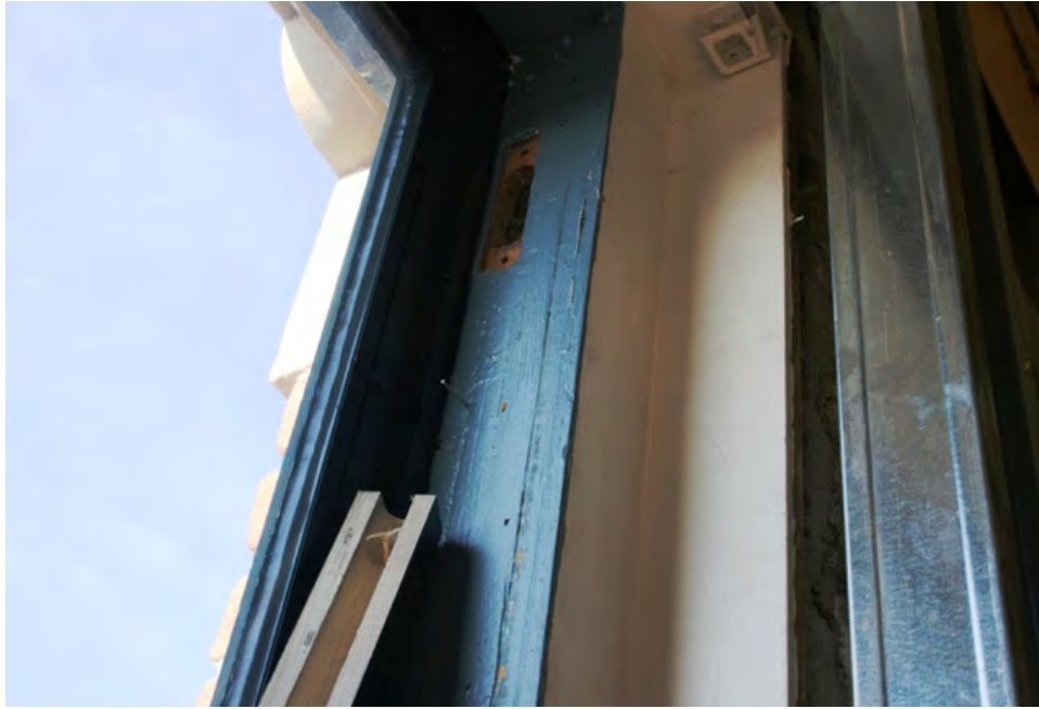
Image 1: Note missing window pulley. A cover, visible at the bottom of the image, was milled to prevent the window from opening fully, to cover the space left by the removed pulley, and to cover the end of the spiral balance.
