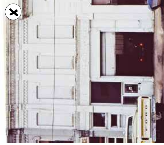
Before rehabilitation: historic windows are missing.
