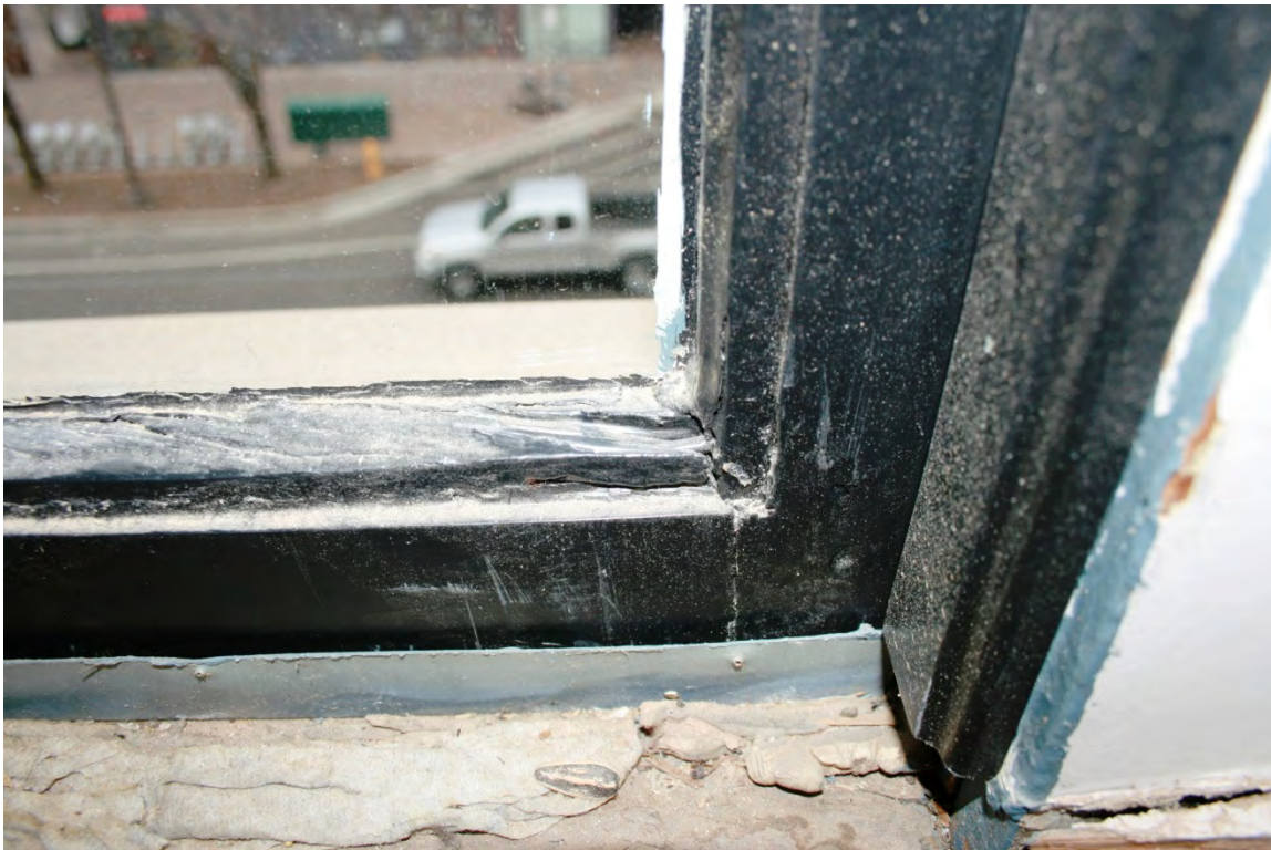
Image 10: Note the condition of the lower rail and the built-up paint
