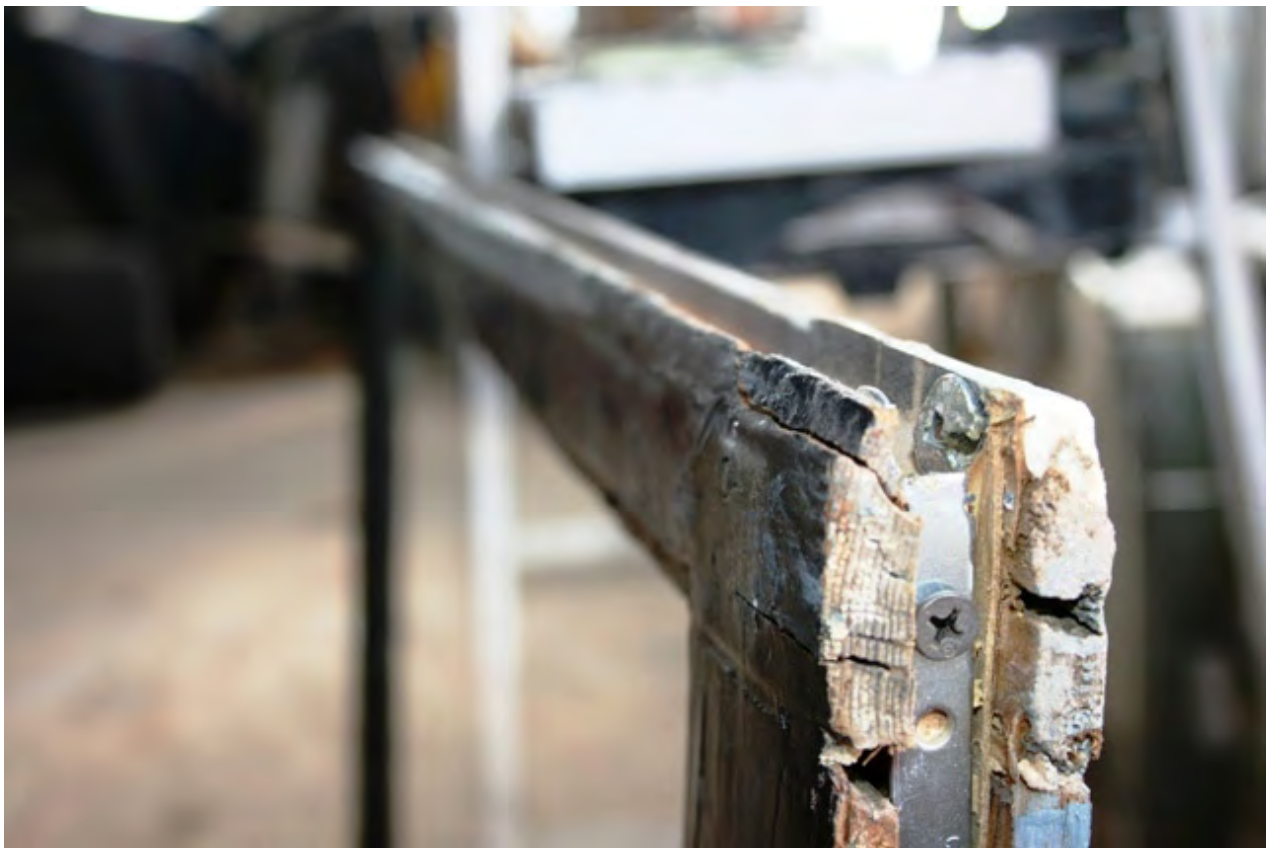
Image 6: Note the split that has already developed as a result of the removal of supporting material. In addition, note the thinly filled epoxy repairs that are adjacent
