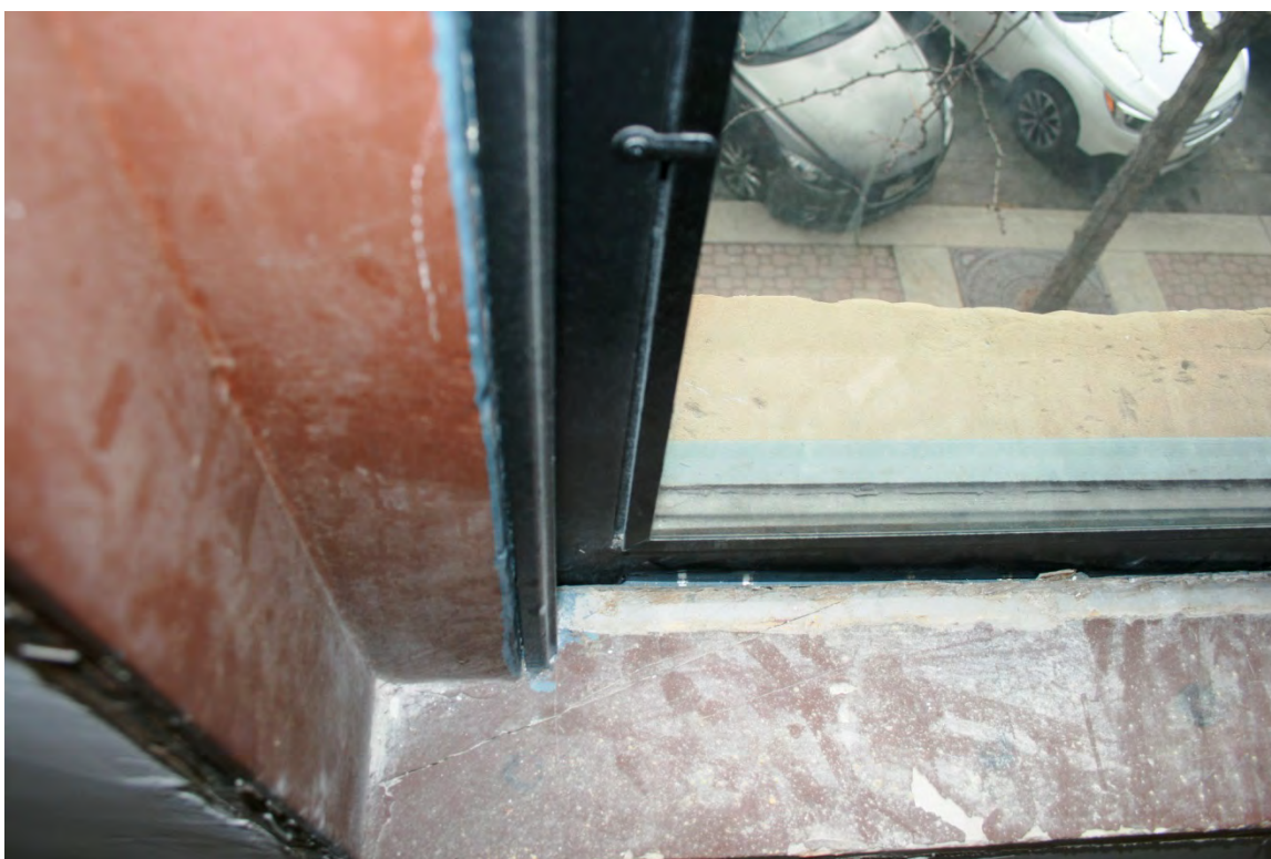
Image 9: Glass panel is slipping. Fit is loose
