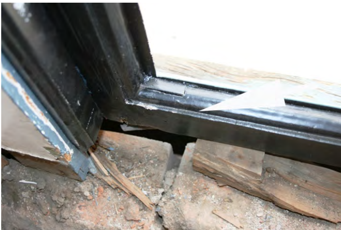
Image 7: Groove cut to house glass panel. The open space underneath the sash is due to the sill and stool being missing, presumably awaiting restoration.
