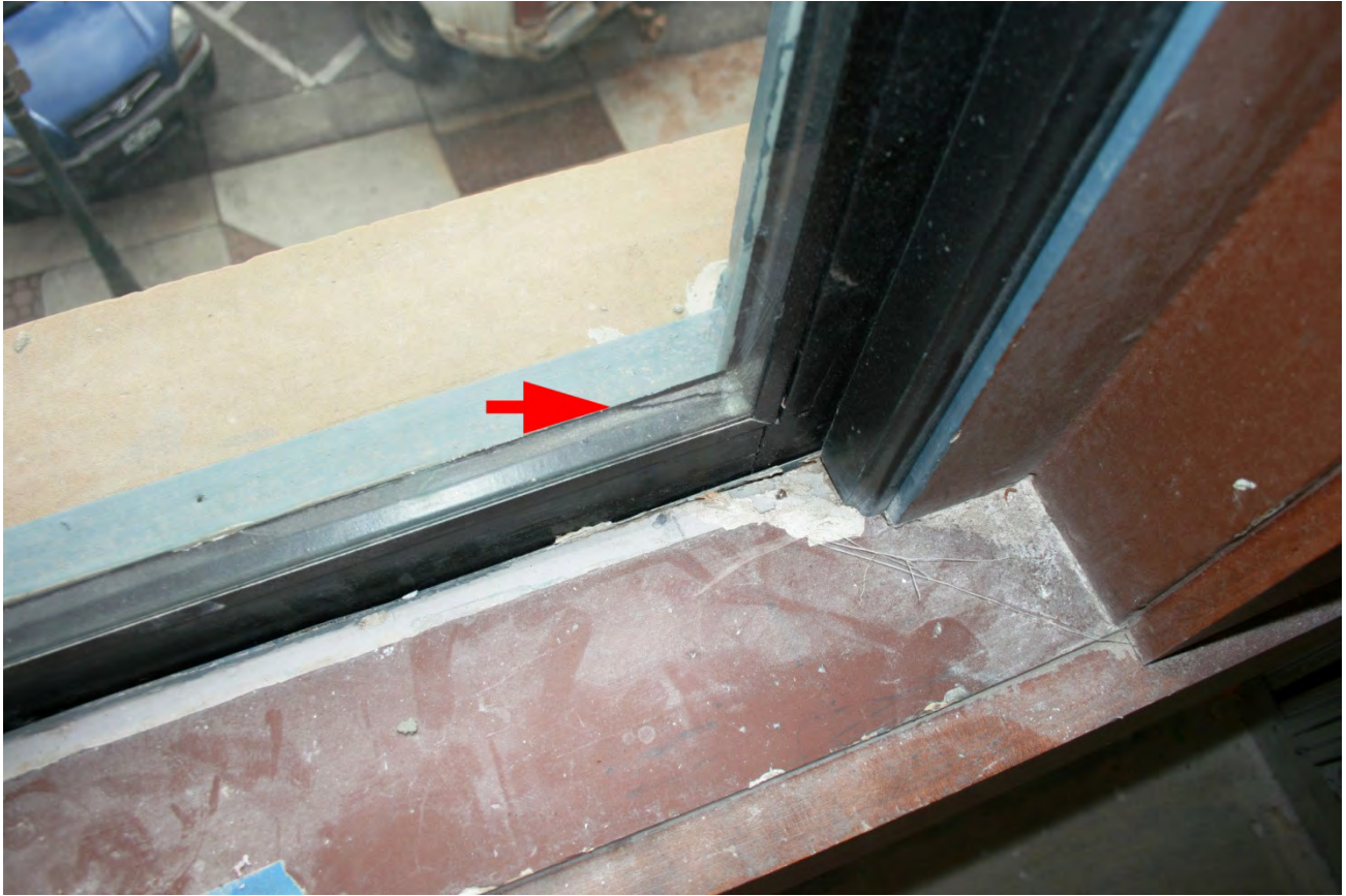
Image 19: Window 002-6, note crack in lower rail
