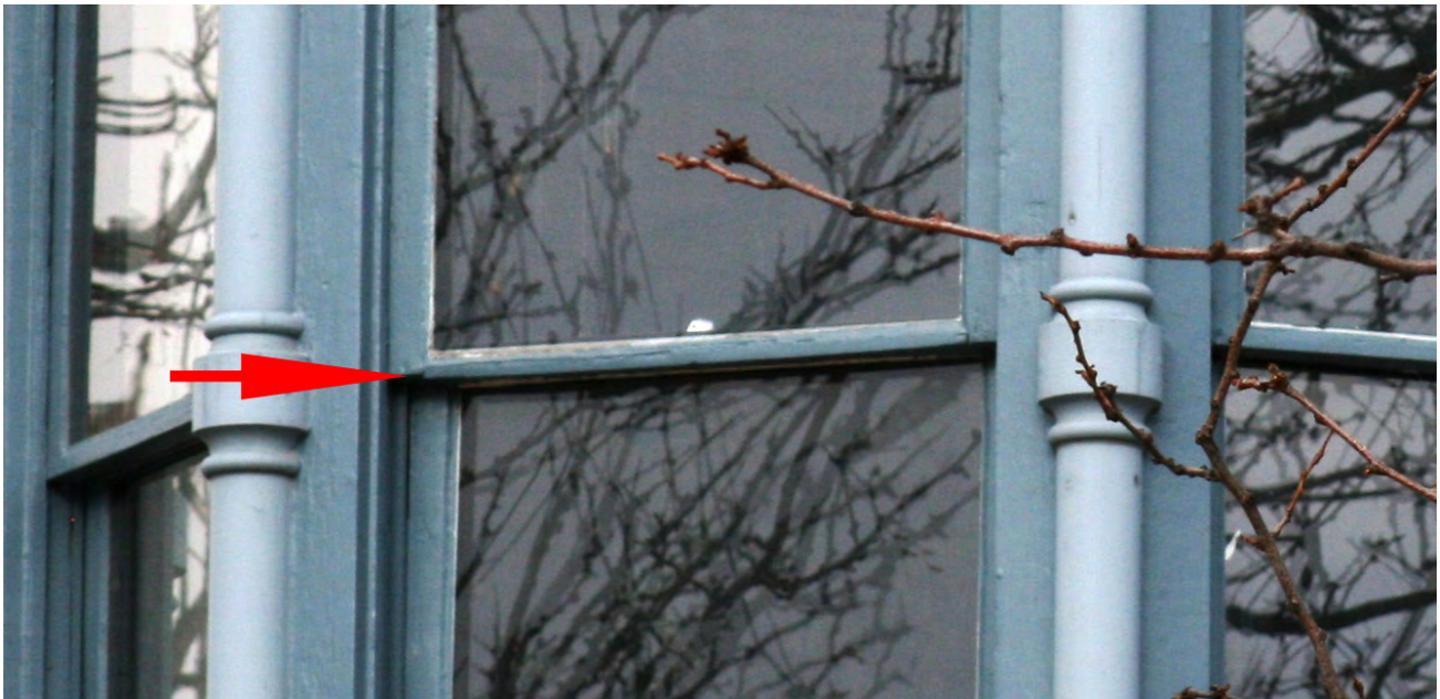
Image 20: Window 002-11, note meeting rail slipping down
