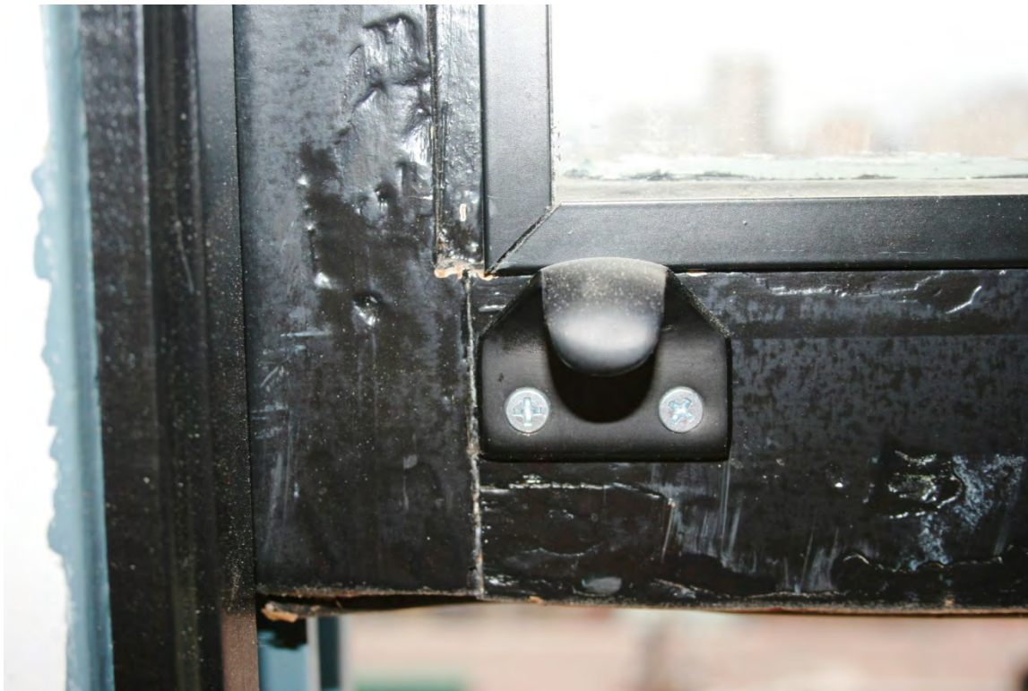
Image 8: Note that glass panel does not fit tight in groove
