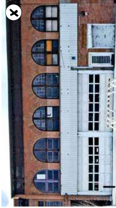
Before rehabilitation: upper story windows in need of repair.
