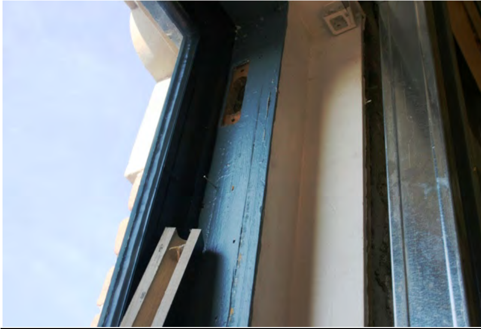
Image 1: Note missing window pulley. A cover, visible at the bottom of the image, was milled to prevent the window from opening fully, to cover the space left by the removed pulley, and to cover the end of the spiral balance.
