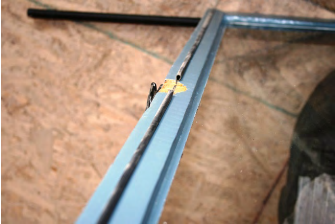
Image 17: Damaged seal at meeting rail
