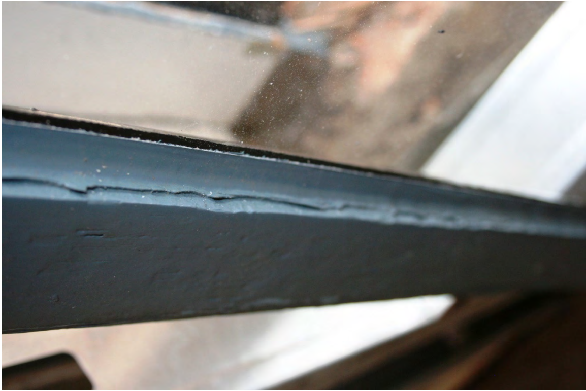
Image 14: Note how the new glazing compound does not come up to the edge of the bed and has a ragged edge
