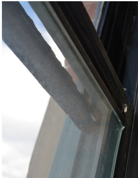
Failing Check Rail
