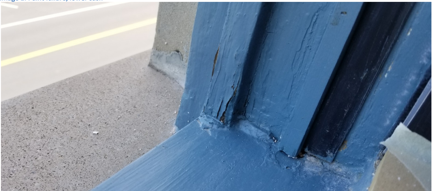
Image 2: Paint failure, blind stop
