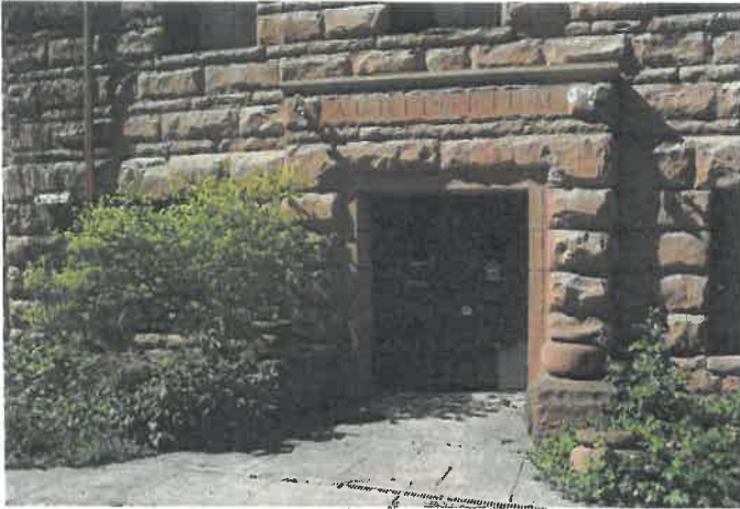
IMPROVE WAYFINDING TO SOUTH ENTRY REPLACE/IMPROVE LIGHTING ADDRESS DRAINAGE ISSUES
