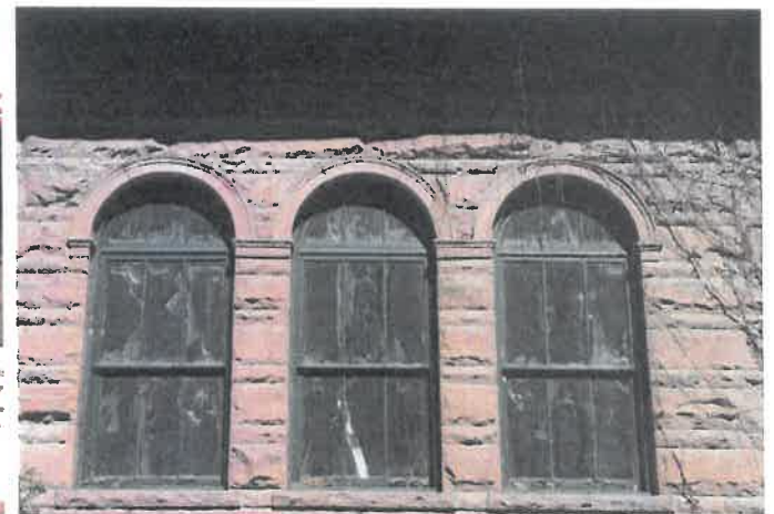
REMOVE PLYWOOD FROM WINDOWS (SHOWN COMPLETED) RENOVATE WINDOWS WITH NEW INSULATED GLAZING REFURBISH WINDOW FRAMES
