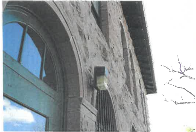
REPLACE EXISTING LIGHTING REFURBISH MASONRY
