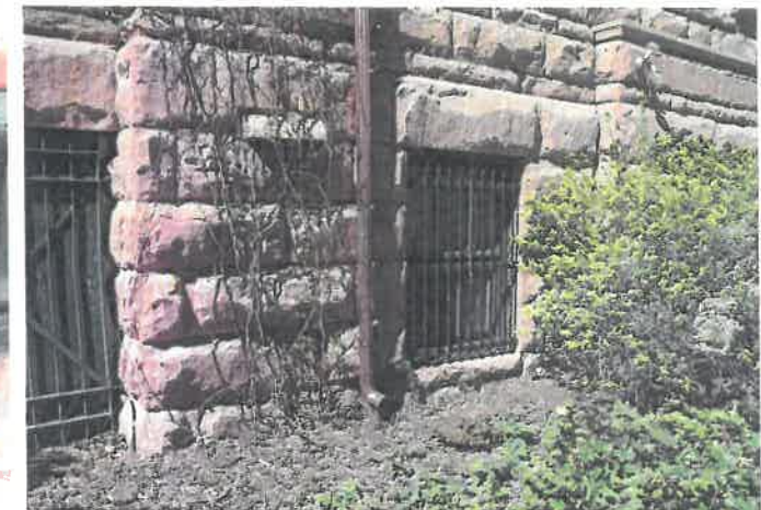
ADDRESS DRAINAGE ISSUES REFURBISH WINDOW FRAMES REMOVE IVY
