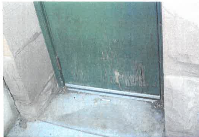
REPLACE DAMAGED EXISTING DOORS
