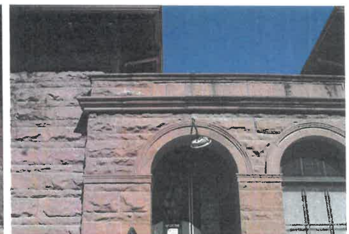
REPLACE/IMPROVE LIGHTING REFURBISH MASONRY
