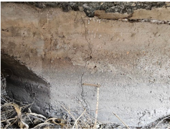
Abutment 2 at north side of widening has medium vertical crack
