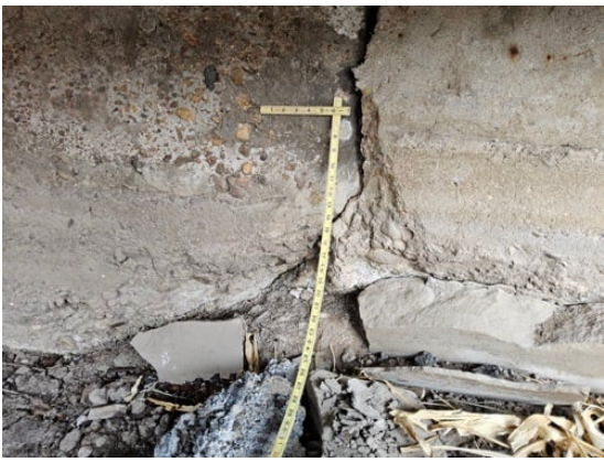
Abutment 2 southeast corner has 0.75 inch wide crack
