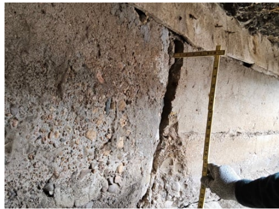
Abutment 2 southeast corner at crack at top is leaning into channel
