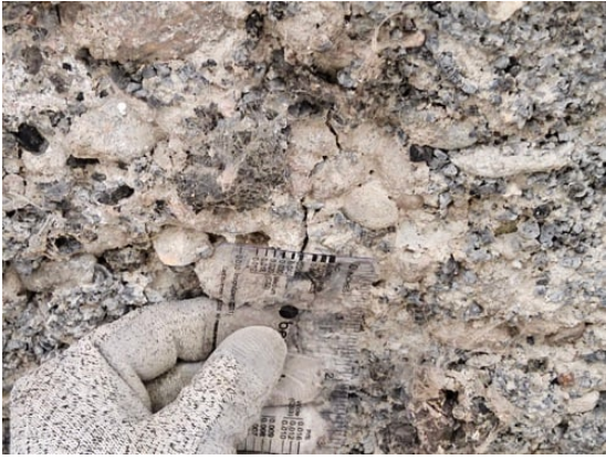
Slab 16 feet from Abutment 1 has medium transverse crack, typical
