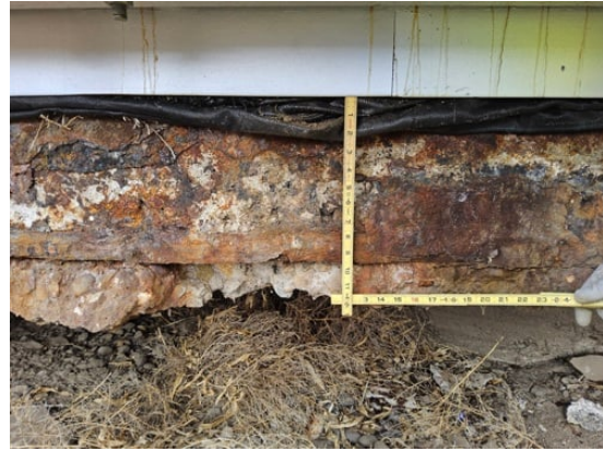
Exterior member at midspan has sag
