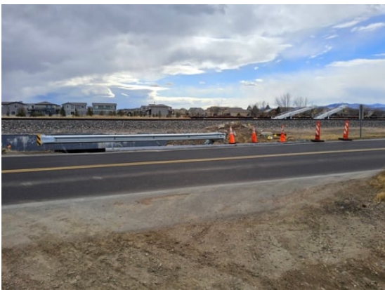
South rail damage looking south
