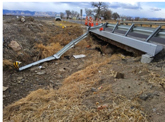
South rail damage looking west
