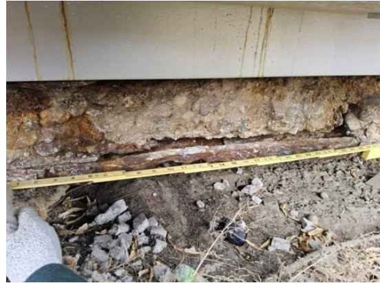
Exterior member has 2 foot section out of plane
