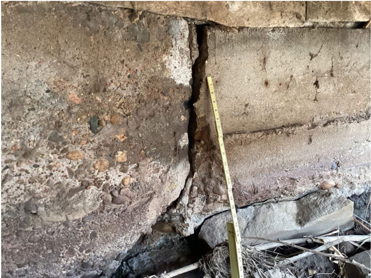
Abutment 2 under widening has wide full height x full depth vertical crack with spalling and abrasion
