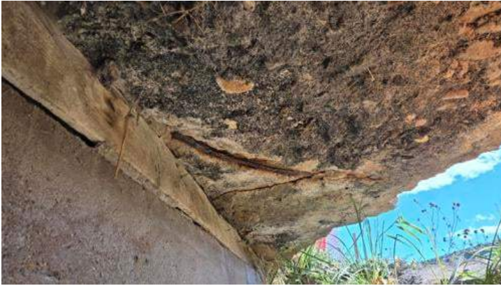
Area of exposed cross bracing shows no intermediate members
