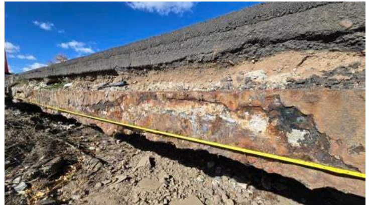
South vertical plate has failed 21 feet 2 inches from Abutment 1
