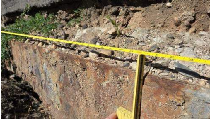
South member at midspan has 1.5 inch sag
