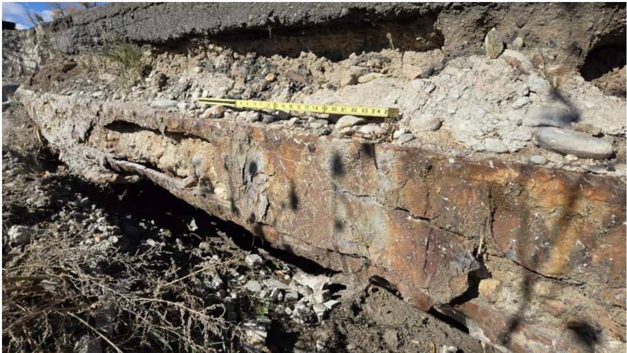
South vertical plate has R4 corrosion with 80-100% section loss
