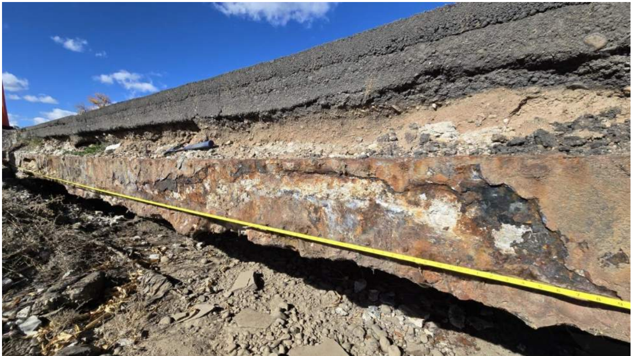
South vertical plate has failed
