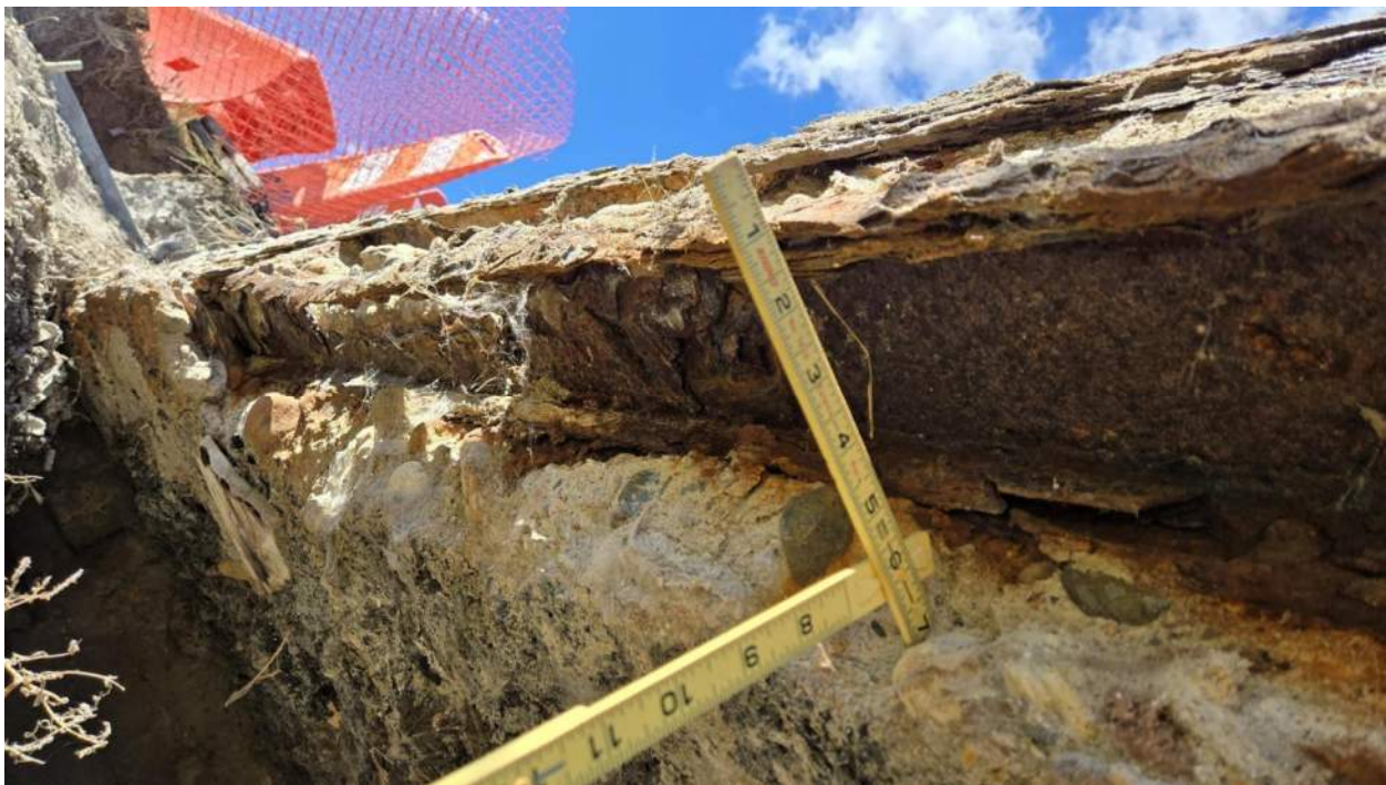
South member bottom channel south flange and web has R4 corrosion with 80-100% section loss
