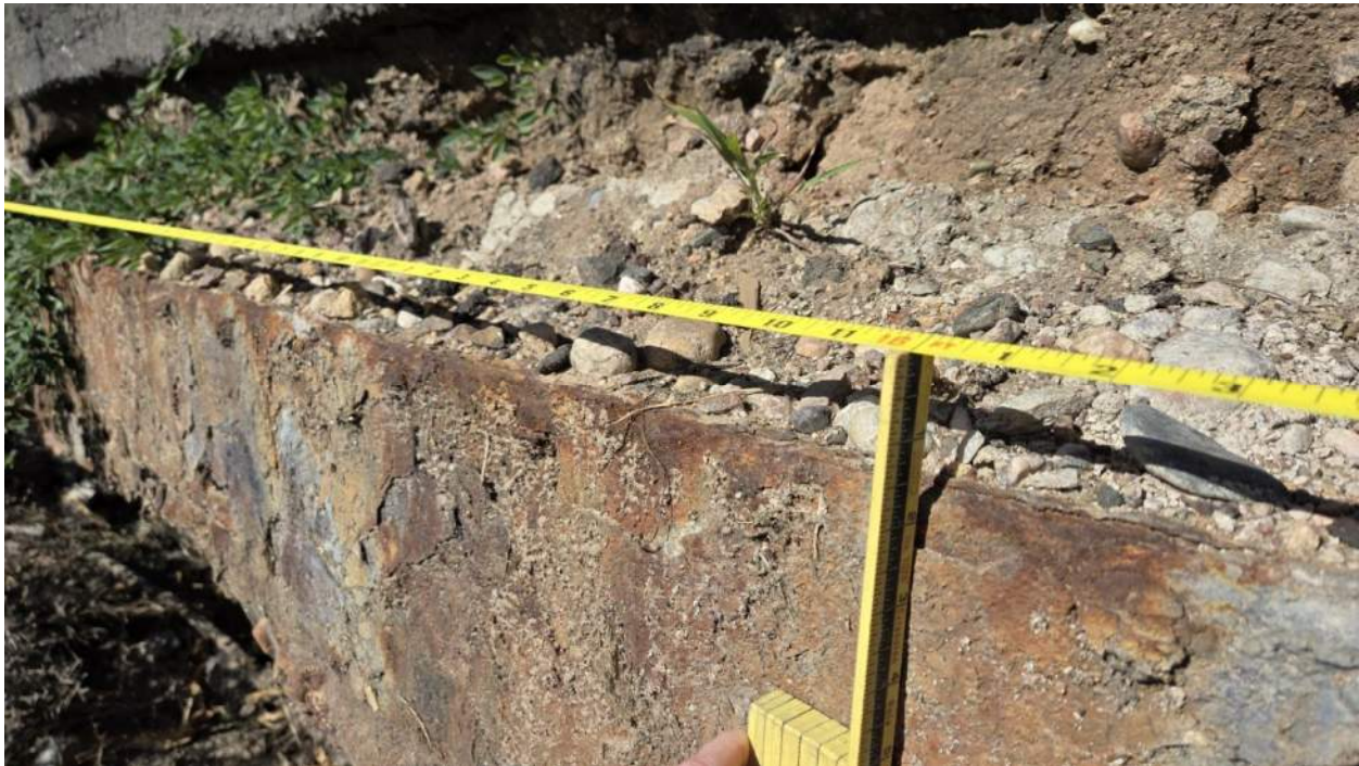
South member at midspan has 1.5 inch sag
