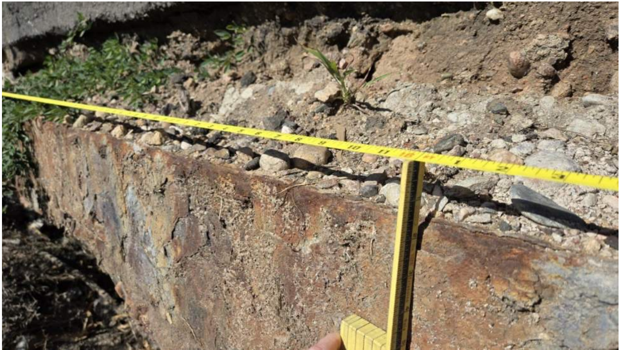
South member at midspan has 1.5 inches vertical sag
