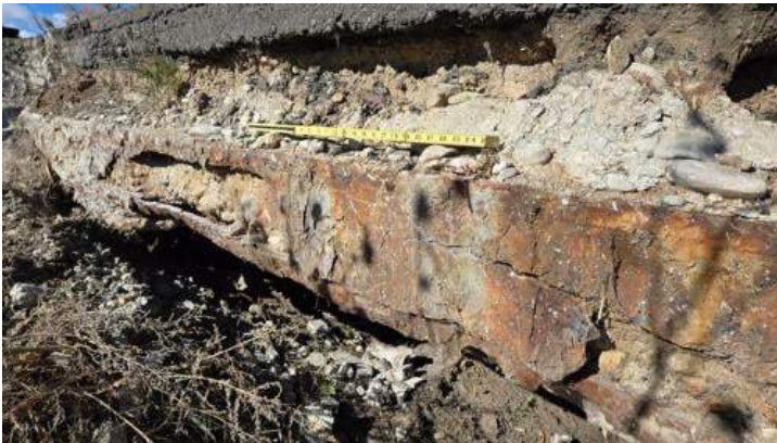
South member 4 feet from Abutment 1 bottom channel south flange and web have 80-100% section loss for 6 feet
