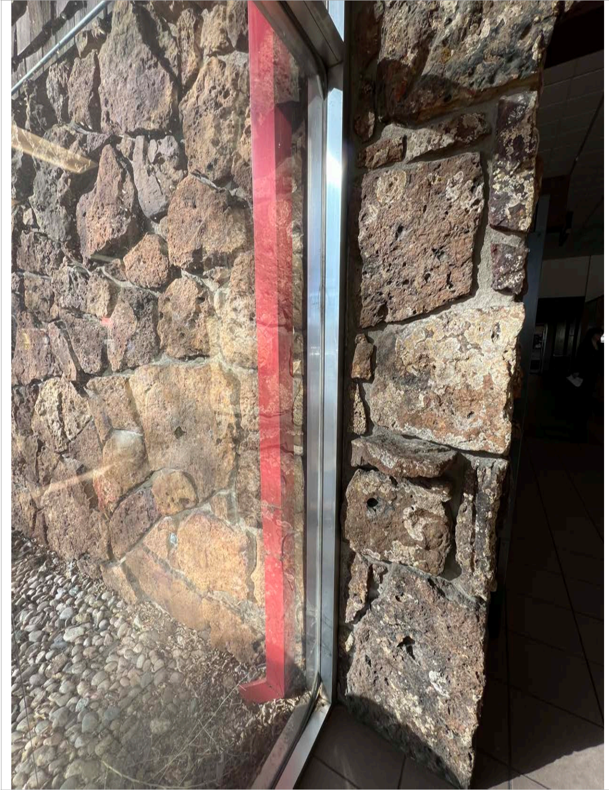
10. East Elevation - Image of connection of aluminum frame, single glaze window with stone veneer. Image courtesy of BEE. 2024.
