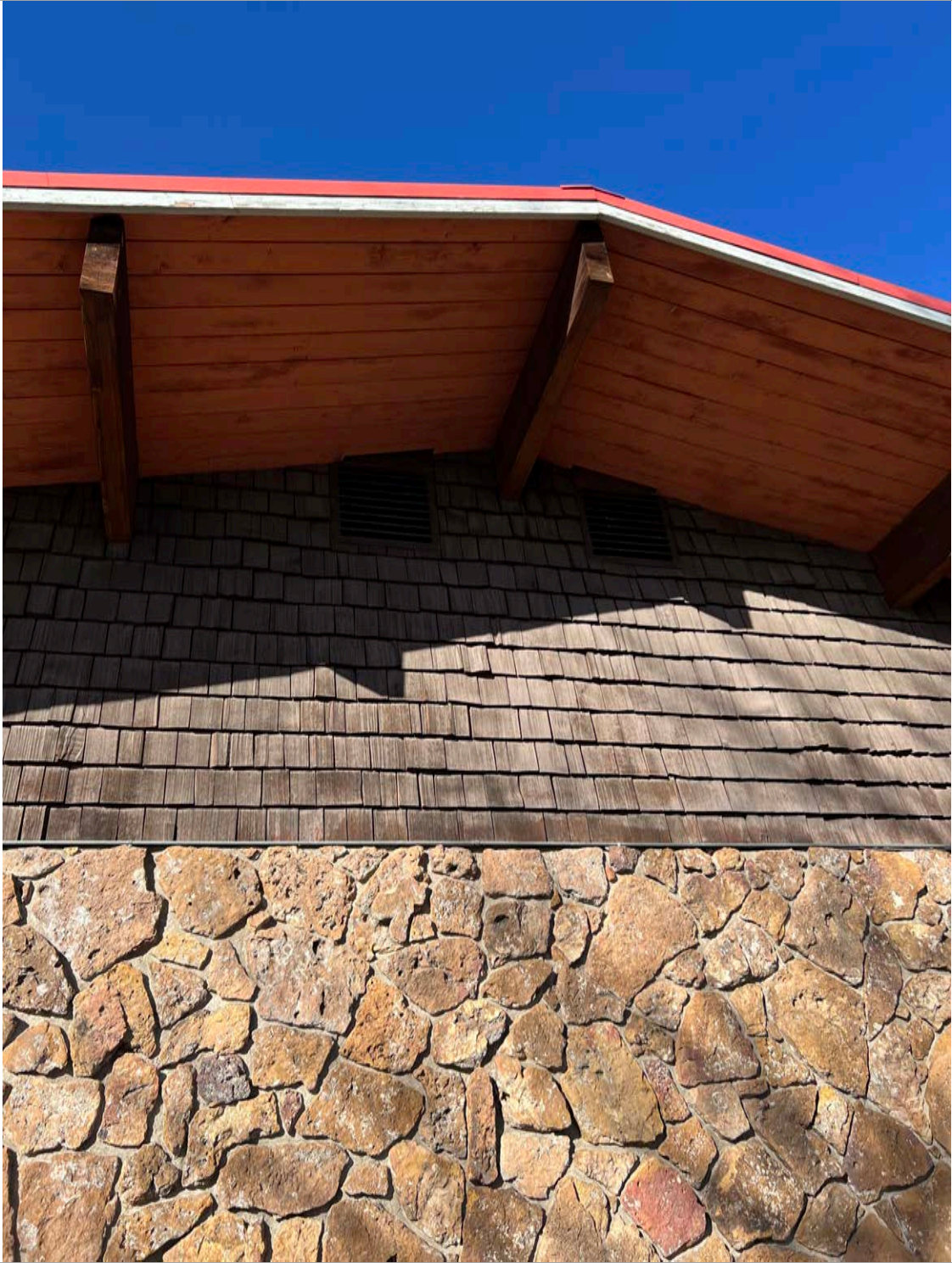
9. East Elevation - South portion, with stone veneer, shingles, exposed rafters and red metal roof trim over fascia. Image courtesy of BEE. 2024.
