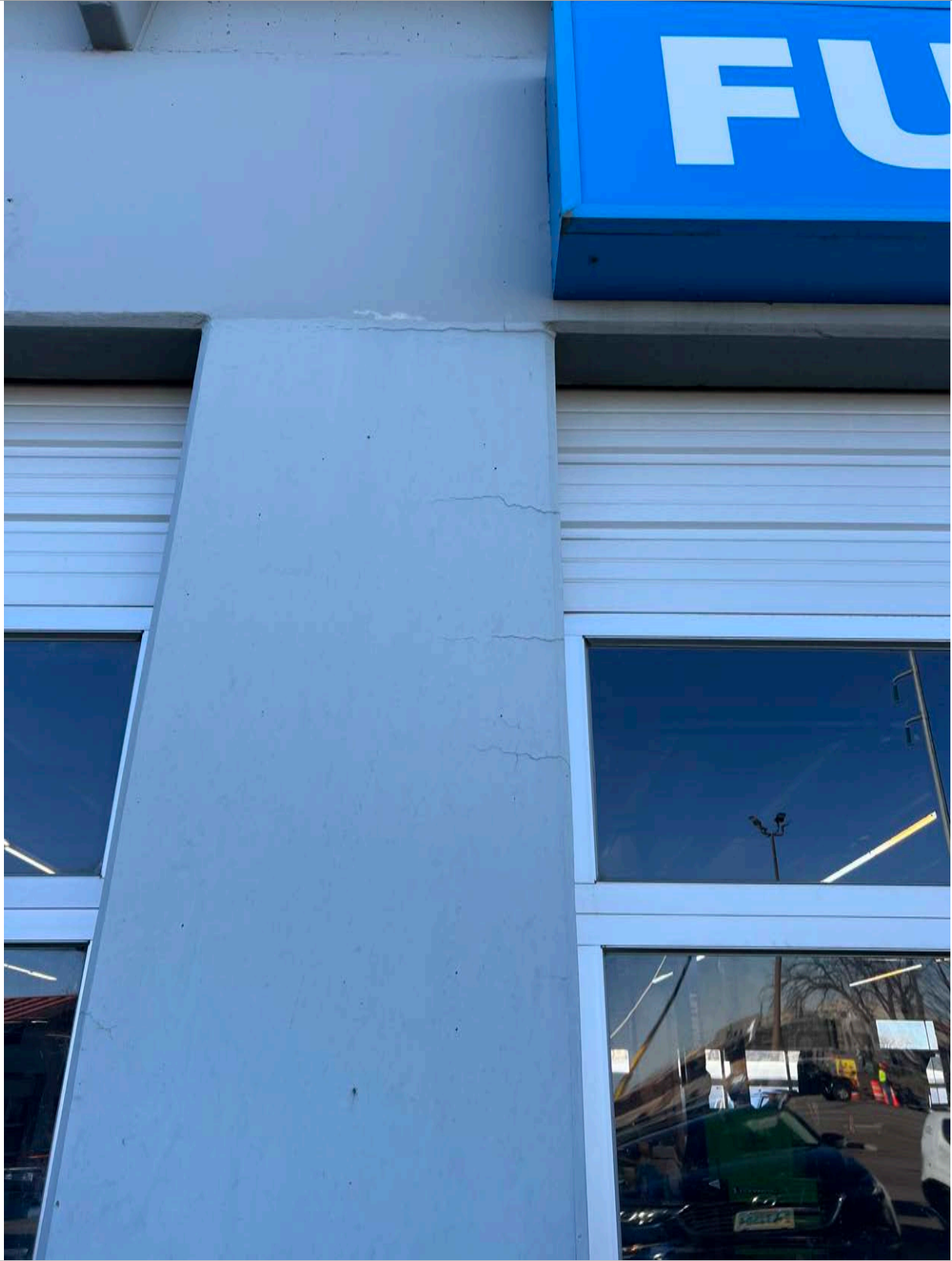
22. North Elevation - Service center, column between bays 2-3. Note the numerous cracks, typical of the columns on both the North and South elevations. Image courtesy of BEE. 2024.
