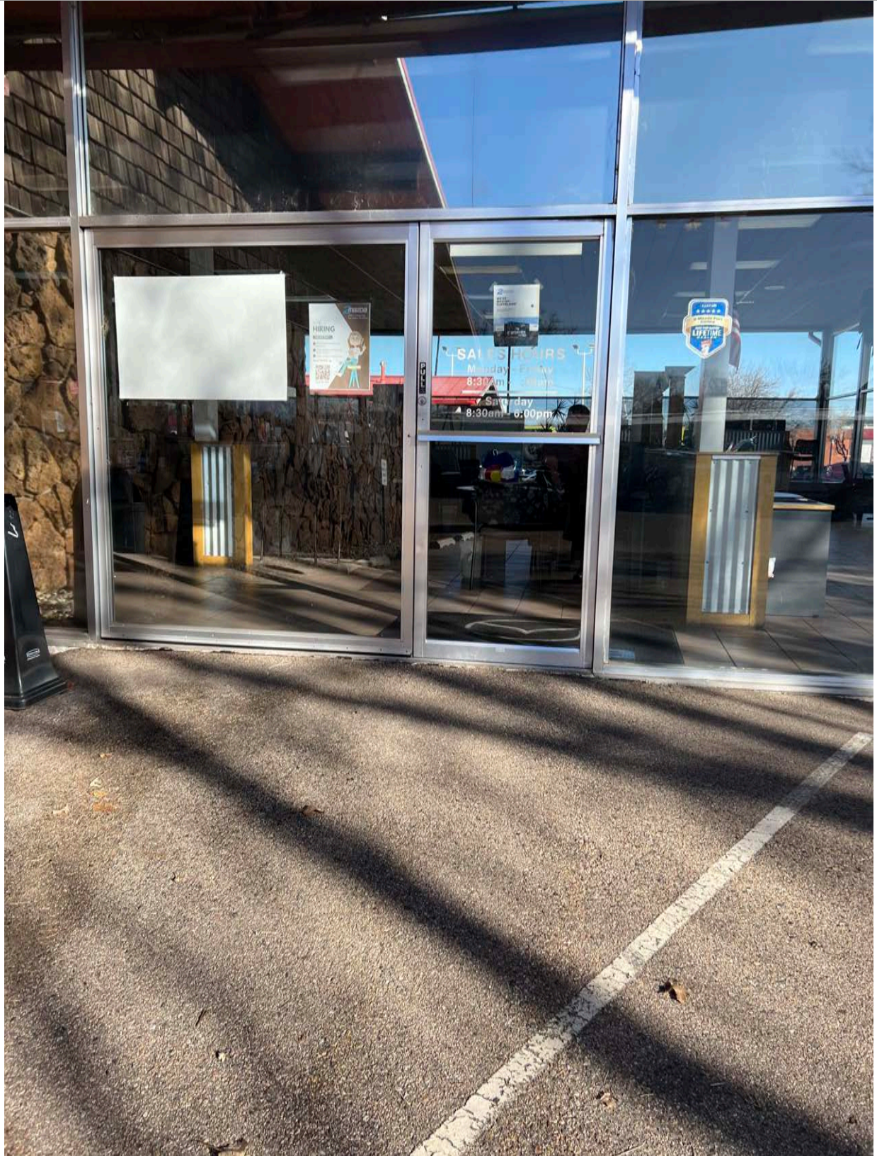
42. South Elevation - Detail of the door and hinged window that open to allow cars into the showroom. Image courtesy of BEE. 2024.
