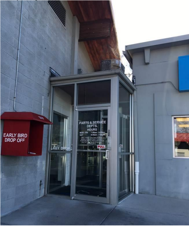
5LR.14283 – Spradley-Barr Parts and Service Entry (Foyer) (Bldg. A) Northern elevation. Looking southwest. December 2017. Image 5LR14283f.
