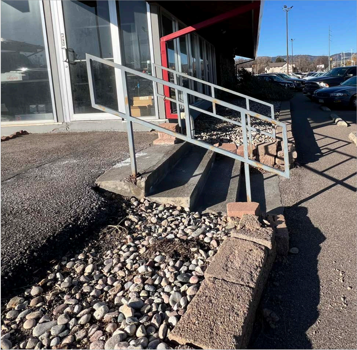
52. Site - Detail of stairs on north side of showroom. Image courtesy of BEE. 2024.
