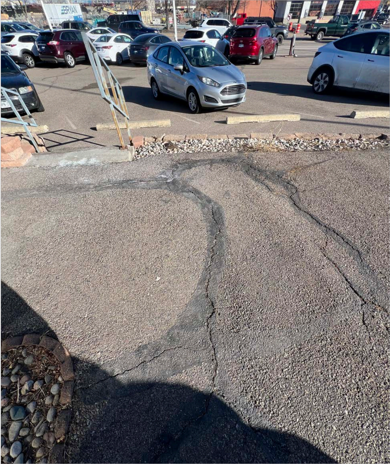
54. Site - Detail of deterioration on east side of Building B. Image courtesy of BEE. 2024.
