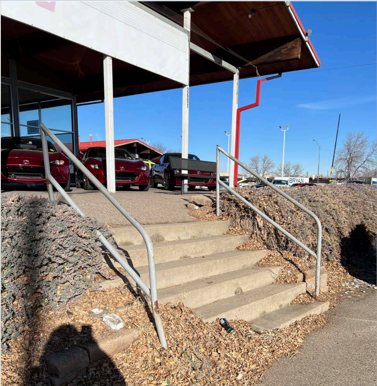
48. Site - Detail of stairs on east side of showroom. Image courtesy of BEE. 2024.
