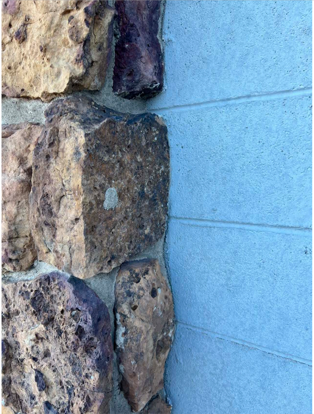
30. West elevation - Detail of stone veneer over CMU. Image courtesy of BEE. 2024.
