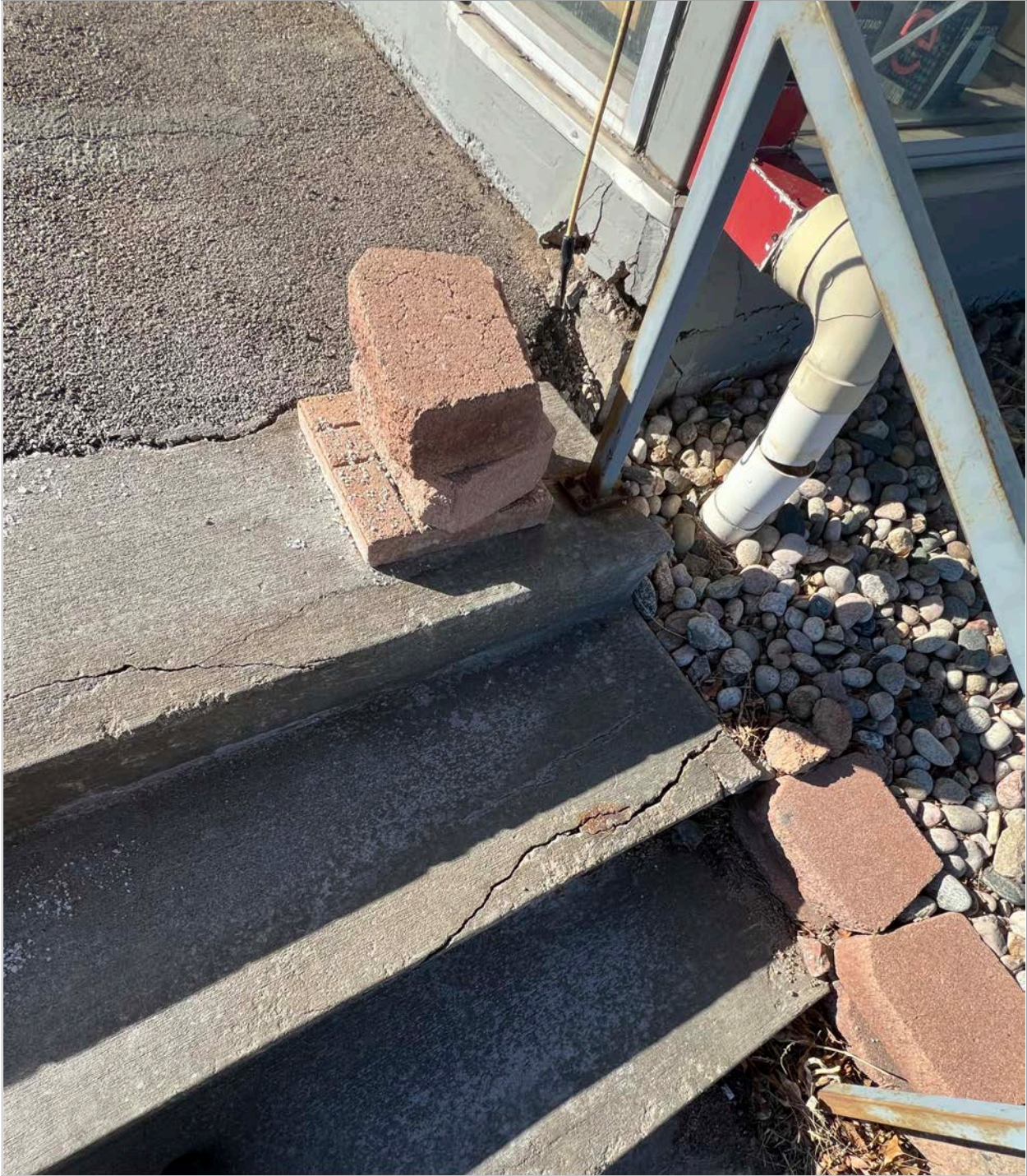
53. Site - Detail of stairs on north side of showroom, showing signs of deterioration. Image courtesy of BEE. 2024.
