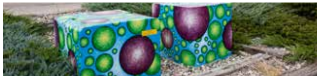
46 painted transformer cabinets
