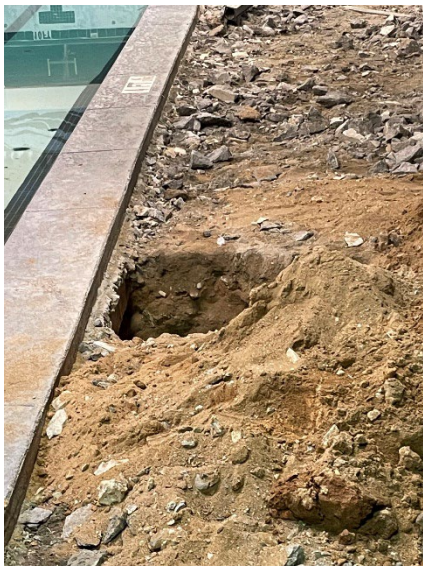
Photo 3: Excavation at inlet pipe leak. View from N. 2/2023
