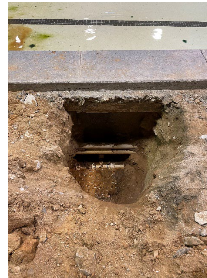
Photo 4: Excavation at inlet pipe leak. View from W. 2/2023
