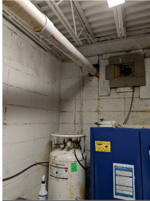
Photo 3 Eastern Basement wall with water infiltration behind equipment
