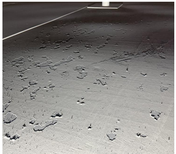
Widespread disbondment observed in large areas of the floor. All edges lifting with poor adhesion. Picture #4
