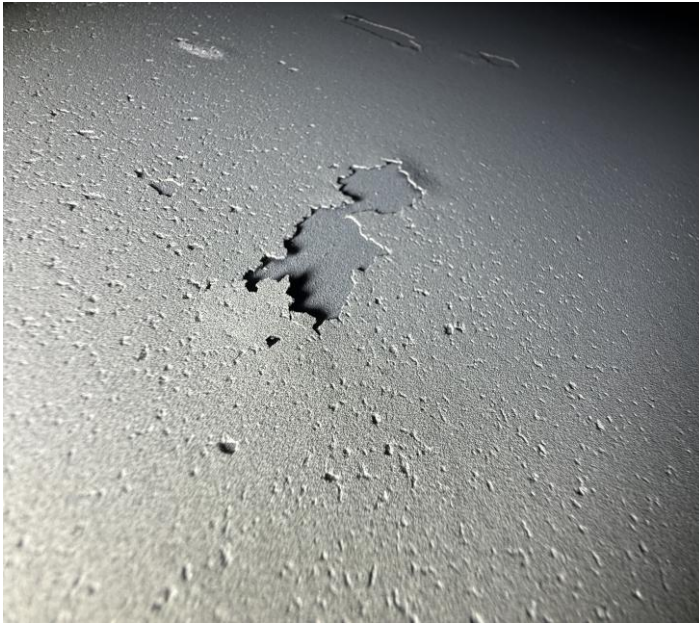
Lifted edges a visible brittleness.
