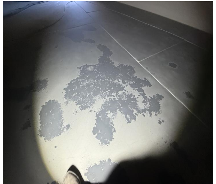
Additional photos of exposed substrate. Picture #2
