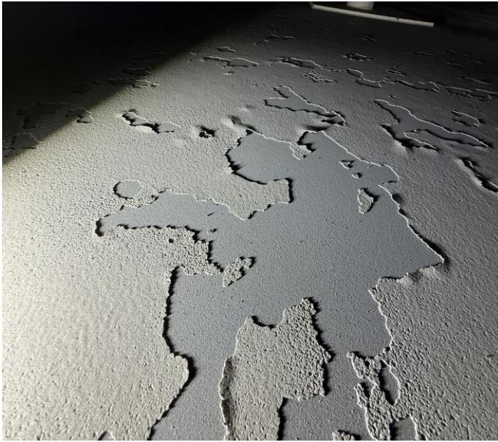
Widespread disbondment observed in large areas of the floor. All edges lifting with poor adhesion. Picture #1
