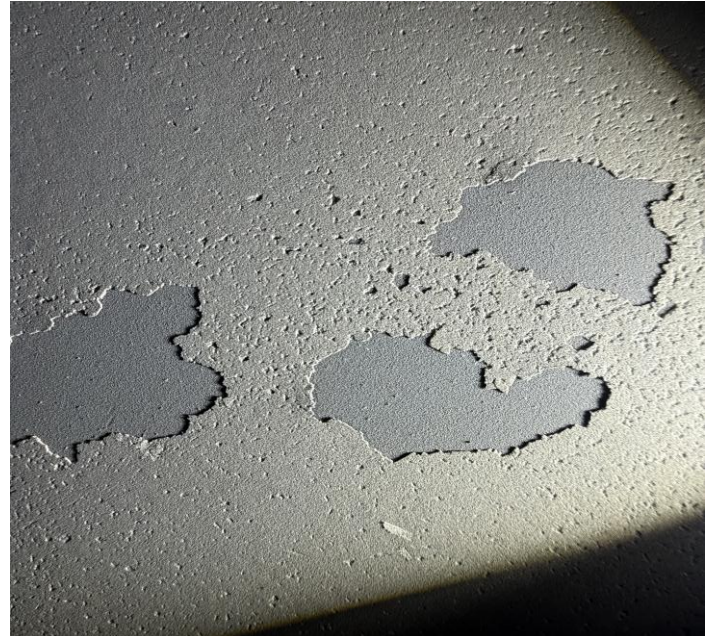
Visible lifting edges and fractures at bare substrate locations.
