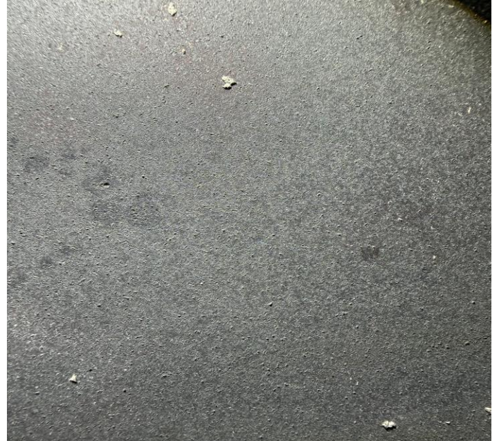
Substrate condition beneath existing coating. Picture #2
