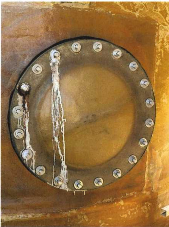
Manway Access Front Face Flange Leak
