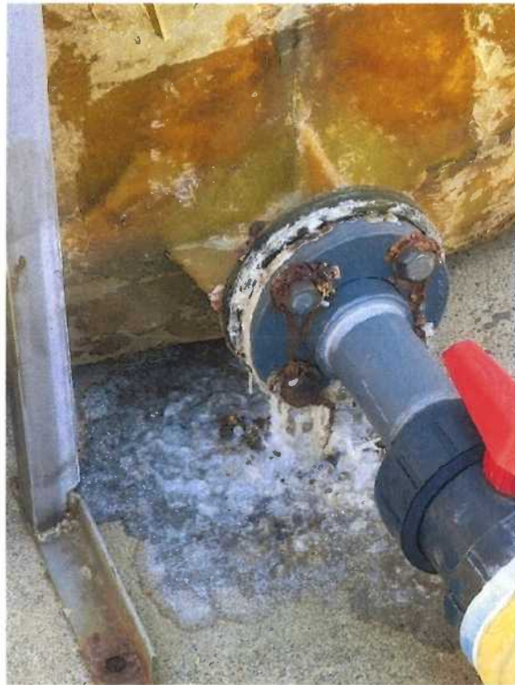
Discharge Front Face Flange Leak (Feed Pumps)
