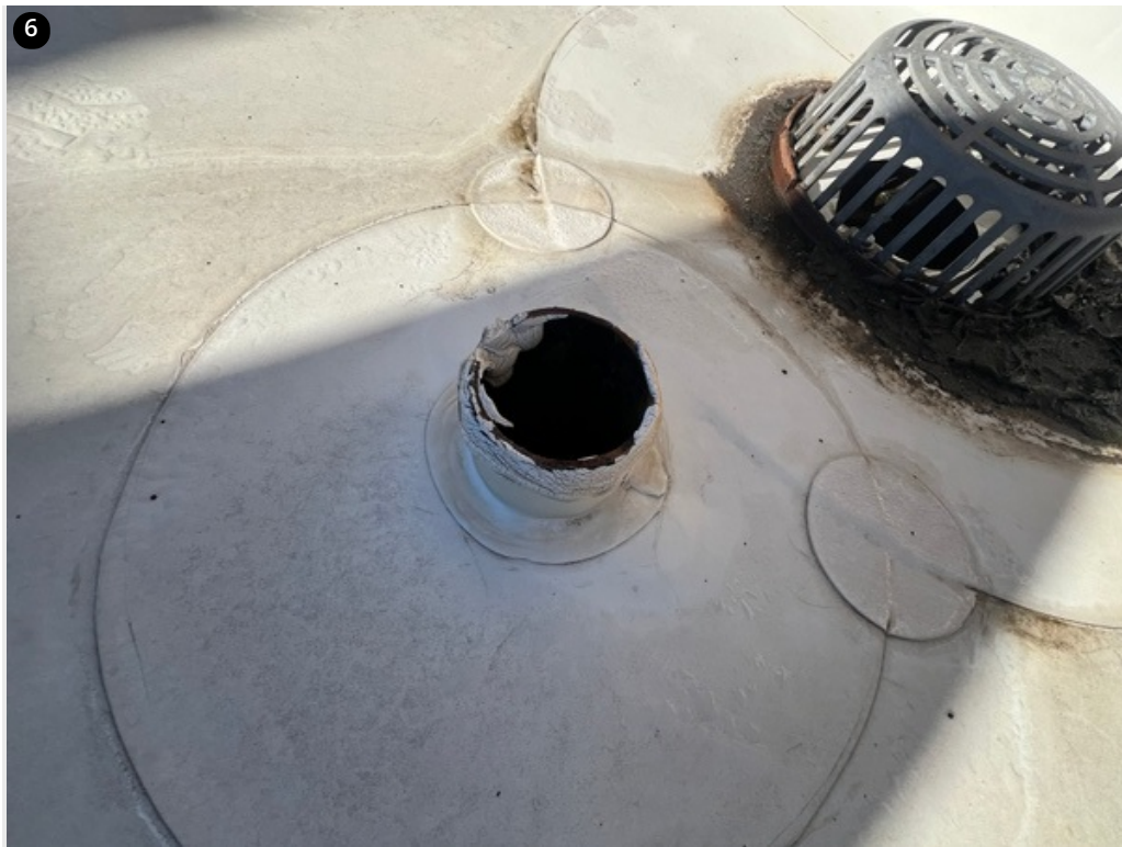
Failed sealant around all penetrations to be removed and sealed.
