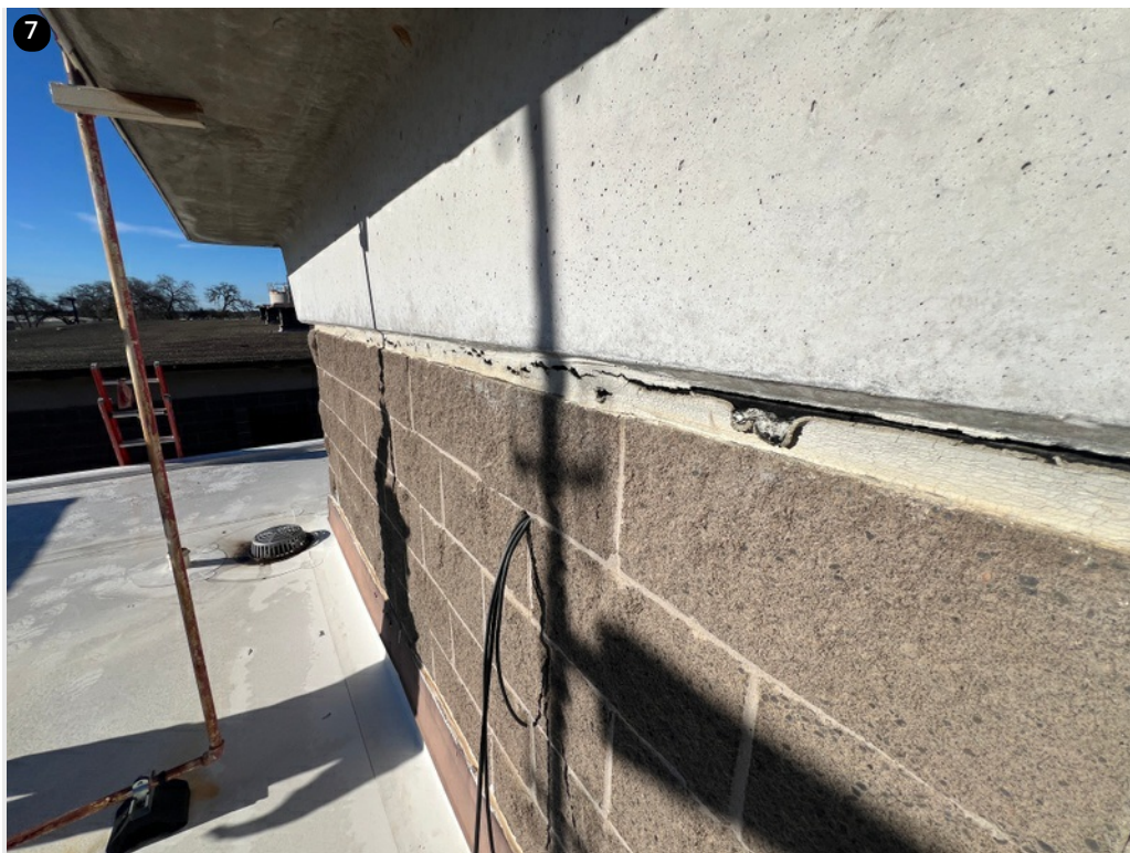
The joint has failed and the backer rod exposed. The failed sealant needs to be removed and replaced.
