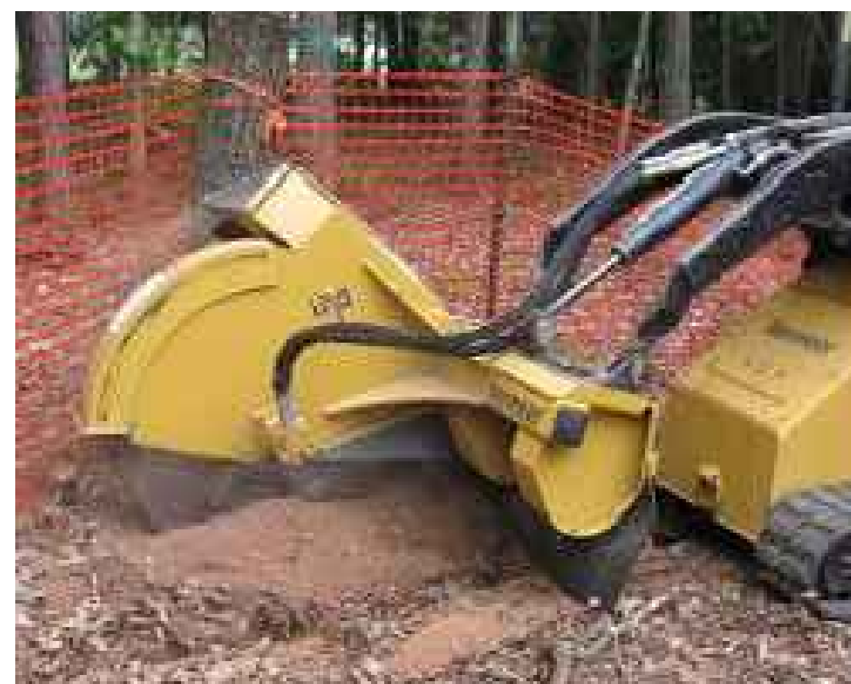
CONTRACTOR TO USE DOSKO OR VERMEER MECHANICAL ROOT PRUNER EQUIPMENT WHEN WITHIN CRITICAL ROOT ZONE OR TREE PROTECTION AREA FOR INSTALLATION OF 4" CONDUITS FOR ELECTRICAL, CABLE, TELECOMMUNICATIONS AND IRRIGATION SERVICES
