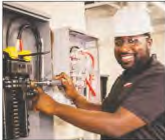
PHOTO PROVIDED A CFK electrical apprentice checks an electrical panel in class on the Upper Keys Center.
