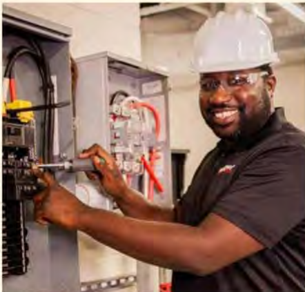
An apprentice checks an electrical panel in class at the Upper Keys Center. CONTRIBUTED
