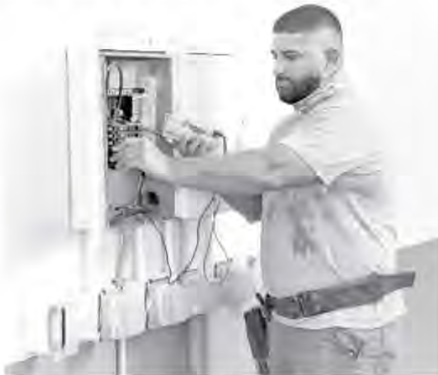
CFK electrical apprentice Donald Chavez Moreno checks an electrical panel. CONTRIBUTED
