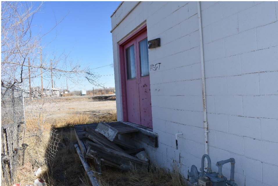
VIEW OF A DILAPIDATED STAIRWAY LOCATED ON THE WEST SIDE OF THE SUBJECT BUILDING
