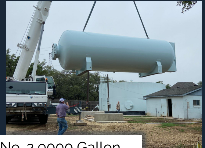
Plant No. 2 9000 Gallon Hydro-pneumatic tank
