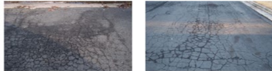
Pavement Condition 11 - 40 (Very Poor/Serious)
