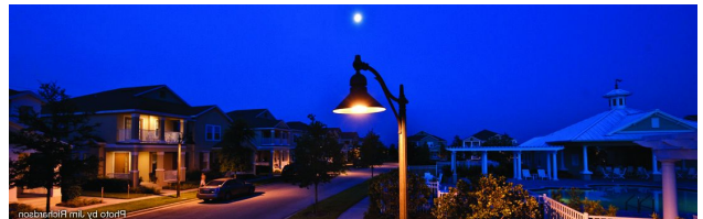
Dark-Sky compliant street light. The fixture is fully-shielded and downward facing with a warm color temperature.
