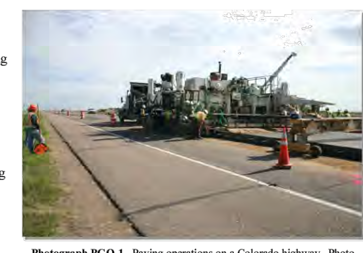
Photograph PGO-1. Paving operations on a Colorado highway. Photo courtesy of CDOT.
