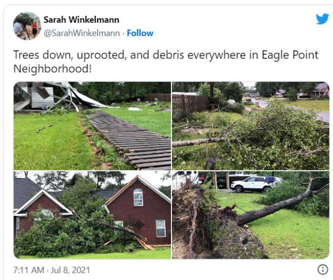
Figure 3-10: Tornado damage from Hurricane Elsa (Winkelmann, 2021).
