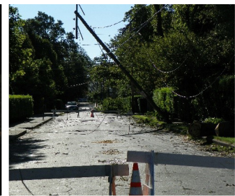
Damage from Tropical Storm Irene
