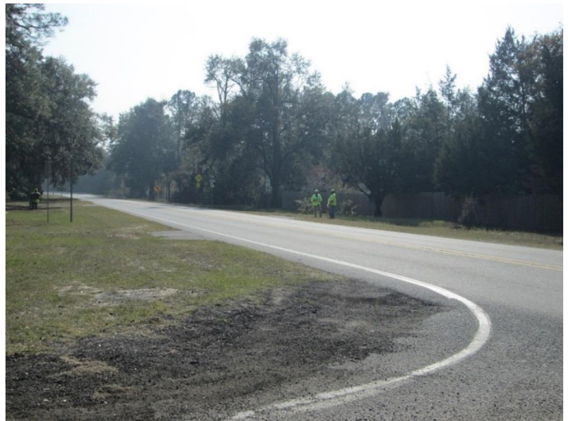
FIGURE 4-21. RUTTING IN THE SOUTHEAST CORNER, FROM VEHICLES TURNING FROM SR 17 ONTO EASTBOUND MARLOW ROAD
