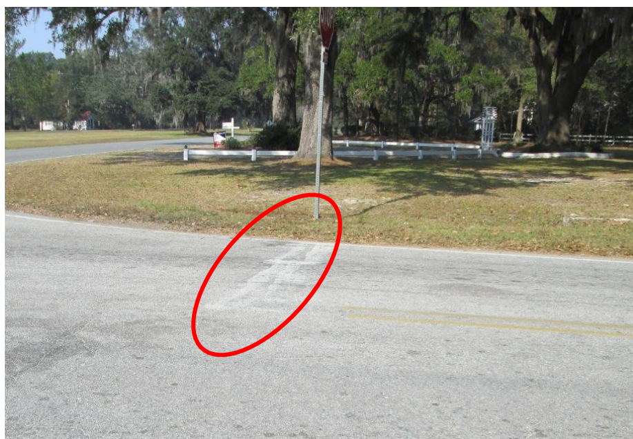
FIGURE 4-6. WORN, FADED STOP BAR AT SANDHILL ROAD AT SANDHILL ROAD/CENTRAL AVENUE INTERSECTION
