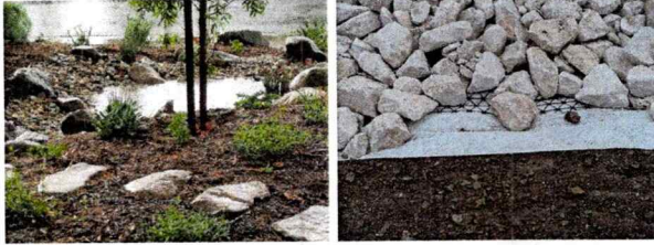
Stone lining the ponding zone of this rain garden. Image credit California Native Plant Society ( https://www.flickr.com/photos/152508454@N05/ )
