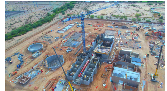
SIGNAL BUTTE WATER TREATMENT PLANT
