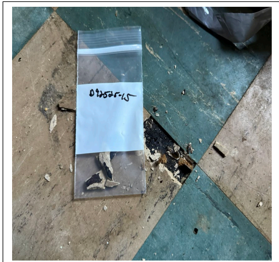
Sample D92525-15: Floor tile positive for asbestos, throughout first floor (Mastic PC less than <1%)
