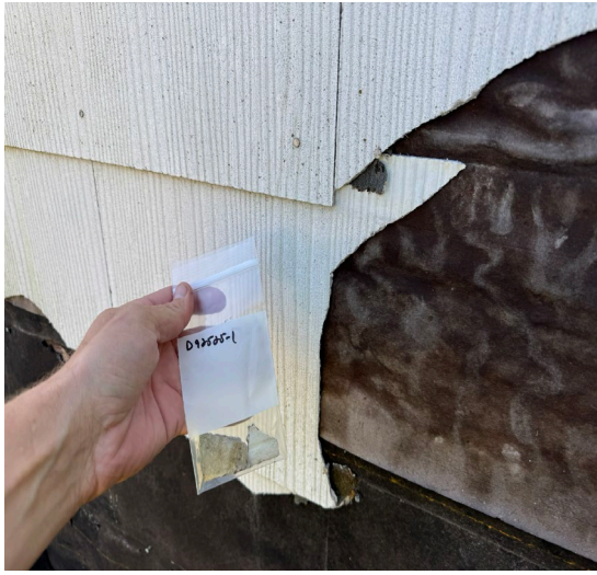
Sample D92525-1: Exterior transite siding positive for asbestos.
