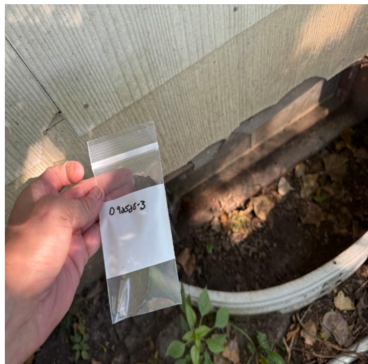
Sample D92525-3: Exterior tar paper behind siding negative for asbestos.
