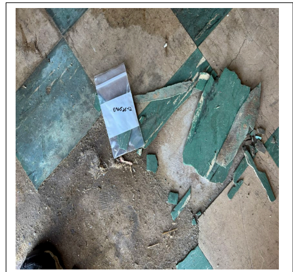
Sample D92525-12: Floor tile positive for asbestos, throughout first floor (Mastic PC less than <1%)
