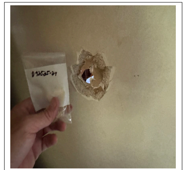
Sample D92525-24: Plaster/drywall backer 2 nd floor West bedroom <1% asbestos. (PC)
