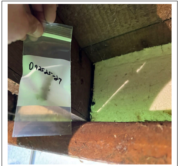
Sample D92525-27: Black caulking in the basement, rim joist, positive for asbestos.
