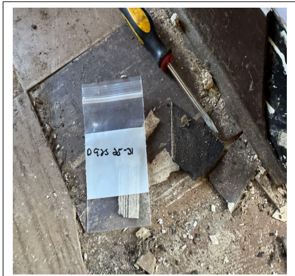
Sample D92525-31: Floor tile 2 nd floor positive for asbestos.
