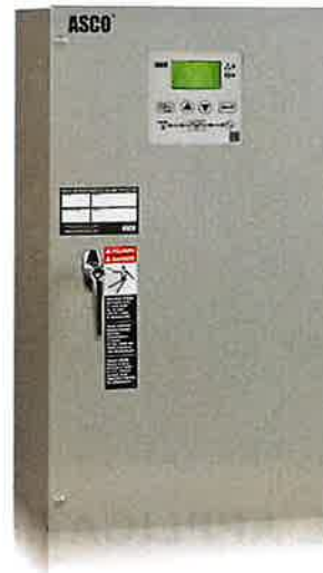
Fig. 1: ASCO Power Transfer Switch rated 200 Amps
