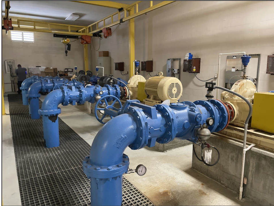
Figure C-1. Hickory Walk WTP High Service Pump Station
