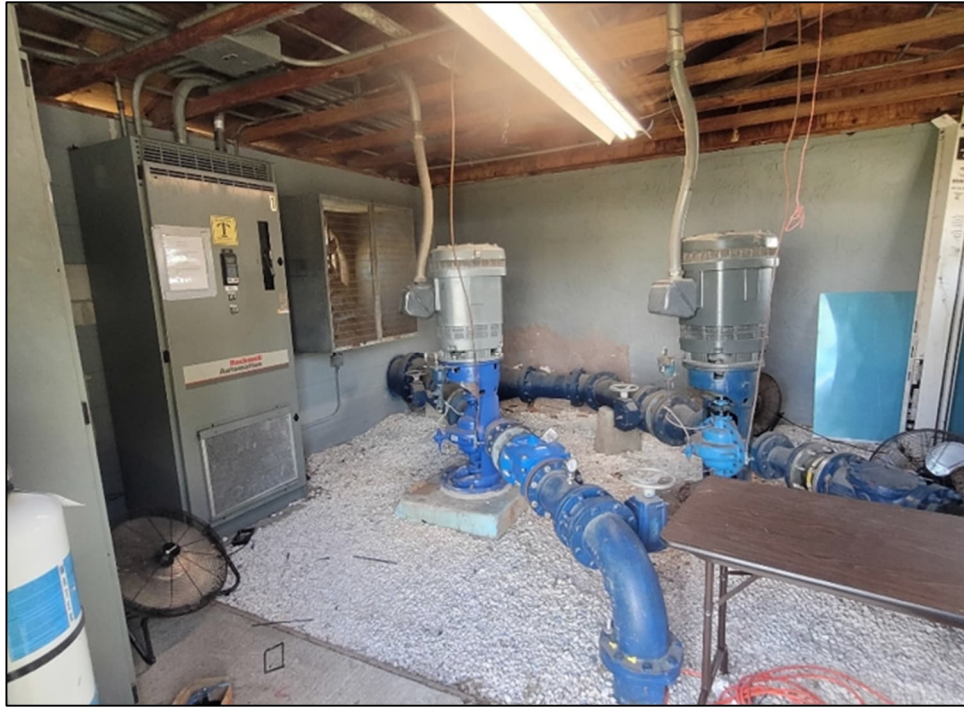
Figure C-3. Riner WTP High Service Pump Station
