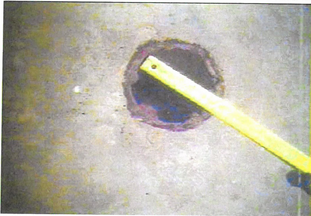
Floor Drain (note rust nodules at perimeter)
