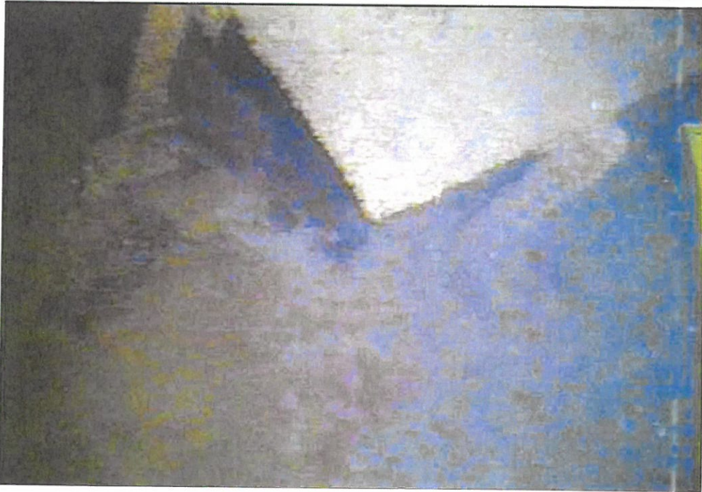
Condition of Outlet and Anti-Vortex Guard (note substantial corrosion)
