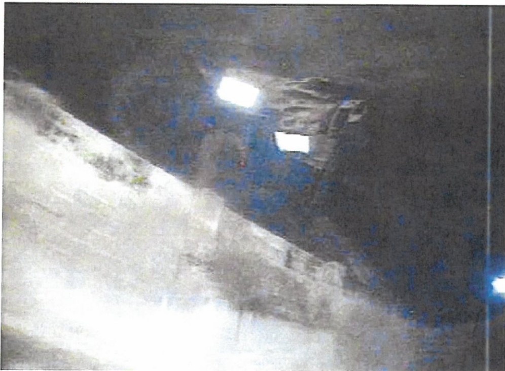
Condition of Baffle Wall and Aerator Ports
