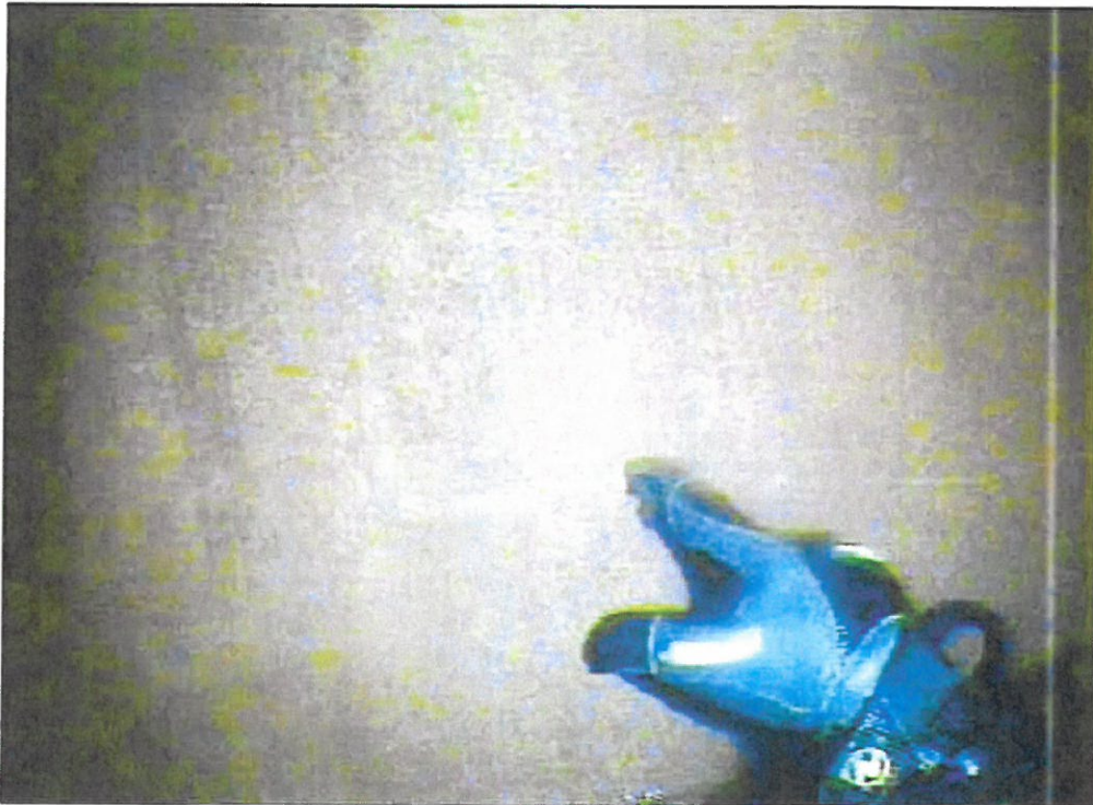
Minor Cracking on Upper Wall
