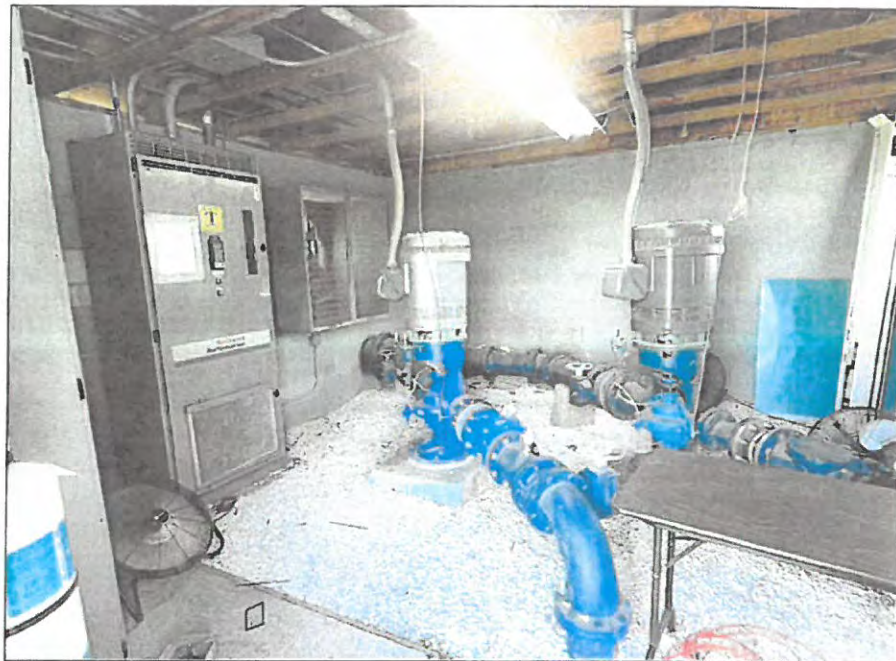
Figure C-3. Riner WTP High Service Pump Station
