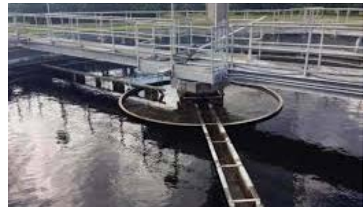
Figure 9. South Regional Water Reclamation Plant
