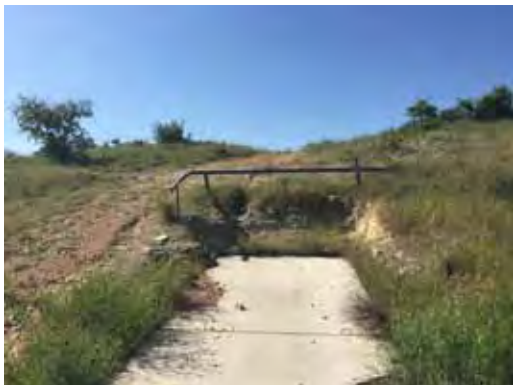
Exterior - Damaged Concrete Path
