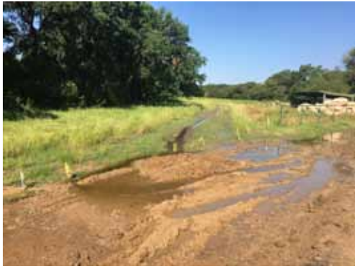
Exterior - Drainage Issues at Park Road
