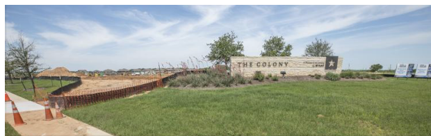
The Colony under construction near Sam Houston Drive and FM 969 outside Bastrop.
