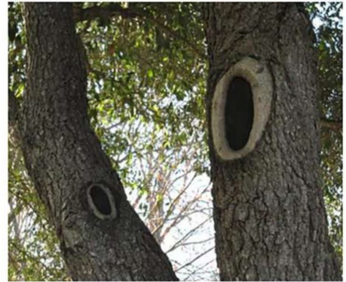
Photo 3. Example of an improper flush cut that should not be performed (image not taken from site).
