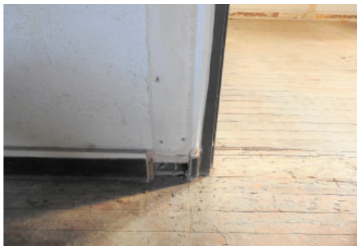
Figure 3.36: Damaged original 1"x6" wood base
