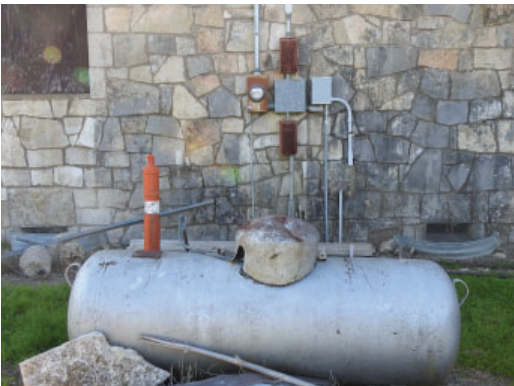
Figure 3.51: West side of building at the edge of the property. Note MEP equipment.
