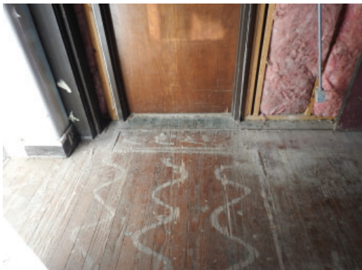
Figure 3.38: Remnants of carpet glue on original wood flooring
