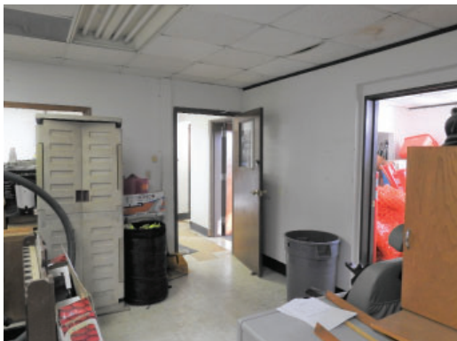
Figure 3.41: Occupied space. Note non-original VCT tile flooring, dropped ACT ceiling, and furred-out wall
