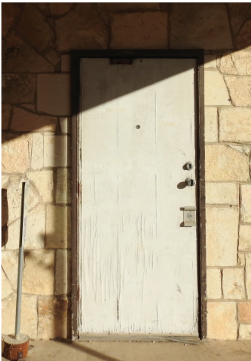
Figure 3.23: Non-original wood door in non-original masonry opening
