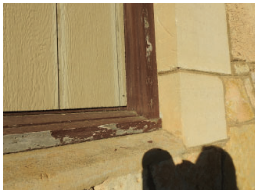
Figure 3.15: Loose paint on window frame assembly
