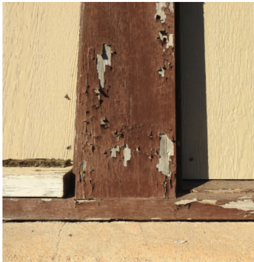
Figure 3.14: Loose paint on window frame assembly
