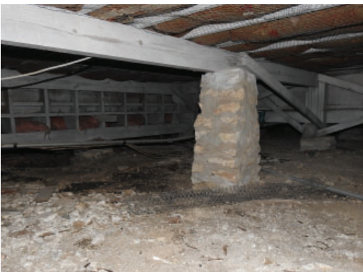
Figure 3.3: Limestone masonry foundation pier and wood beam structure in crawl space under stage at north end
