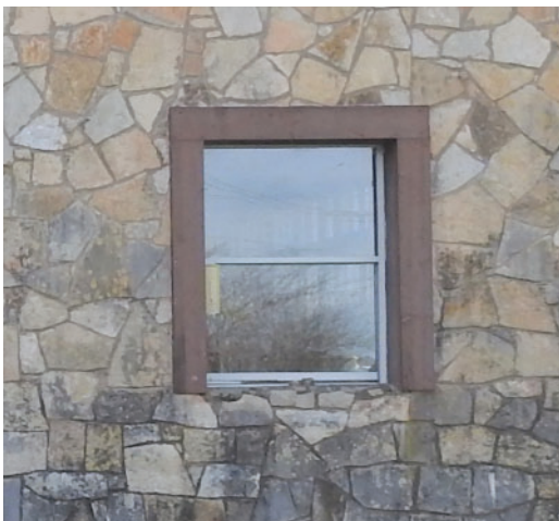
Figure 3.18: Non-original aluminum window on north elevation
