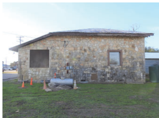
Figure 3.7: North elevation, note biological growth
