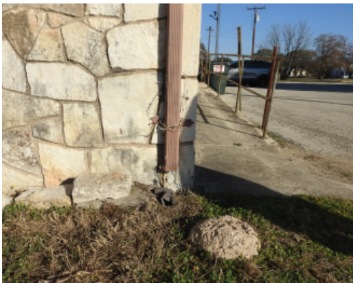
Figure 3.32: Gutter at southeast corner, note missing spout
