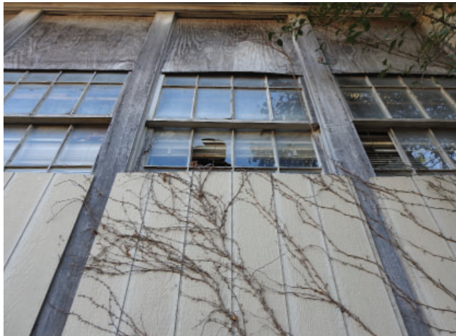
Figure 3.20: Windows have multiple broken lites and vegetative growth
