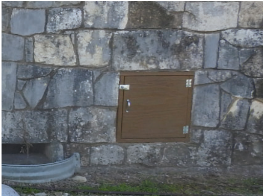
Figure 3.1: Crawl space access door, note biological growth
