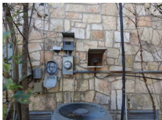
Figure 3.8: Electrical equipment and masonry penetrations at the west elevation
