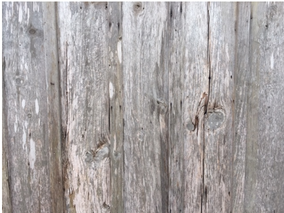
Sealed Weathered Wood Vertical Board and Batten Siding on new Kitchen addition (similar to existing shed out-building)
