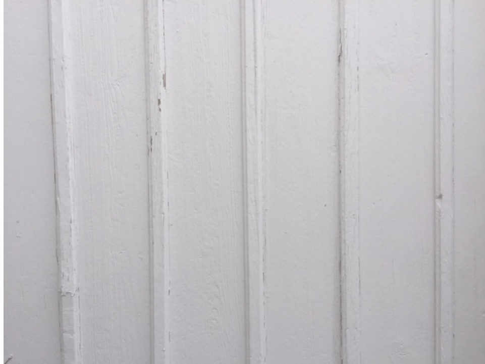
Painted Vertical Board and Batten Siding on new addition to be similar to Short Mama's house (painted White to match)
