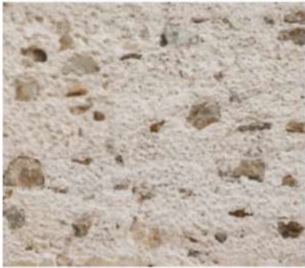
Rubble limestone with heavy mortar smear
