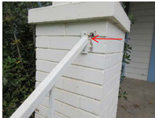
Cracking at patio: Cracking and general settlement was observed at the front patio.
