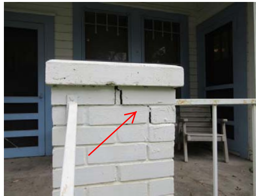
Railing loose: The railing at the front porch is loose.
